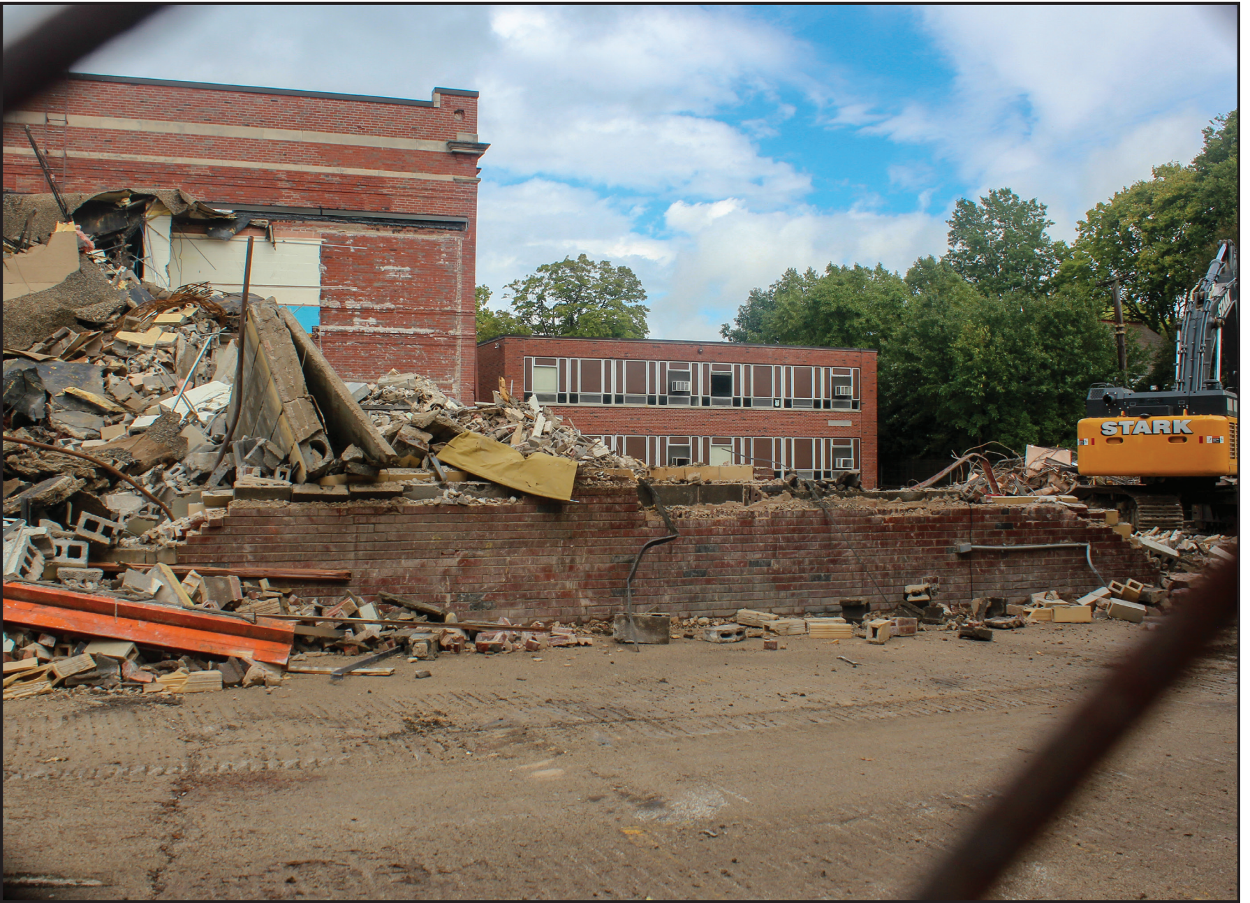
Demolition on Dr Howard. Construction Will Begin on the New Building in Early 2019.
