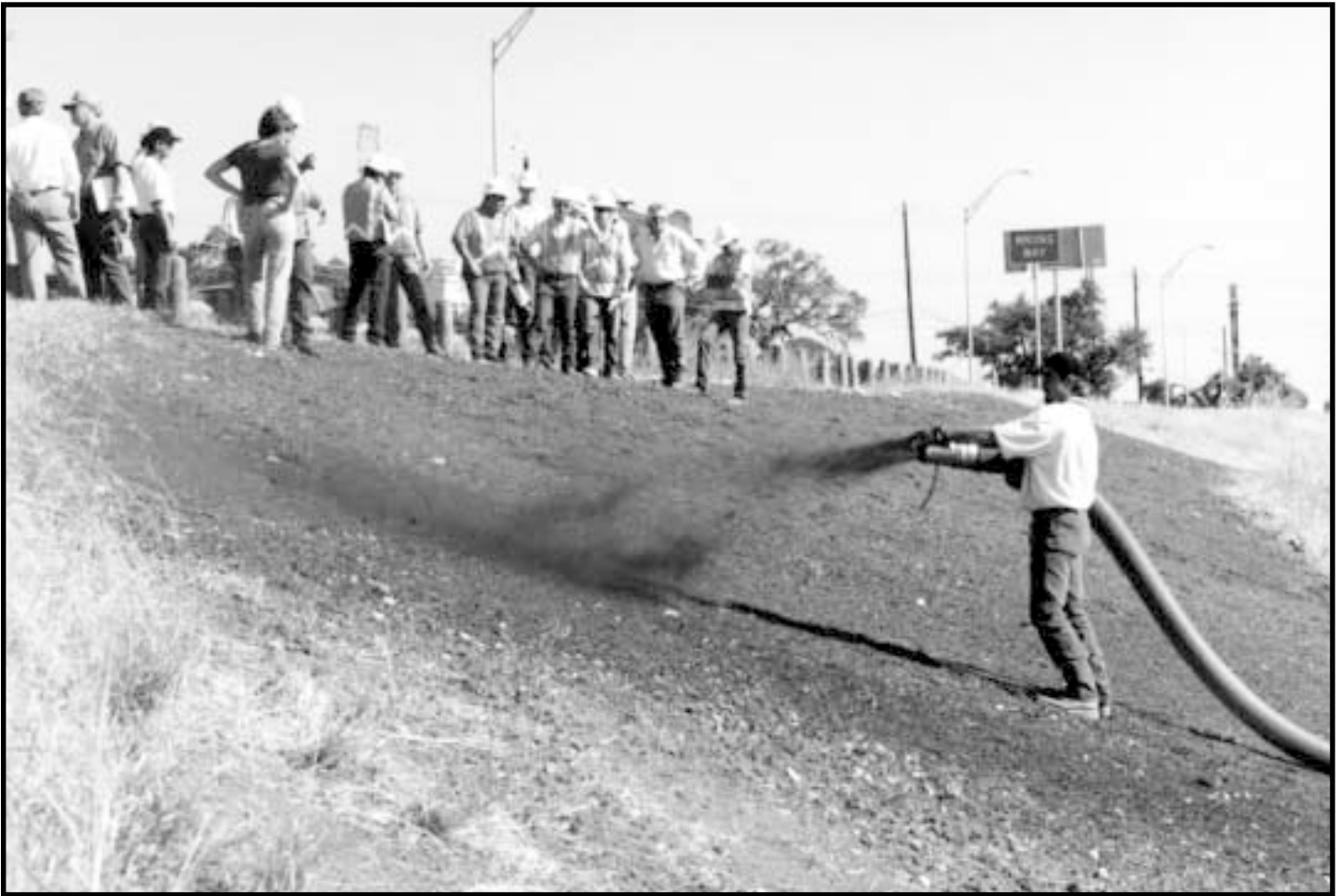
In a demonstration for watching maintenance supervisors, a contractor sprays a manure/wood chip compost mixture on a slope along Loop 1 at Braker Lane in Austin.
