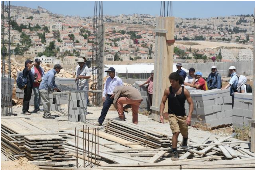
Figure 5. Rebuilding of Atta Jaber home in the West Bank, after being demolished by Israeli army. ICAHD, 2016.
