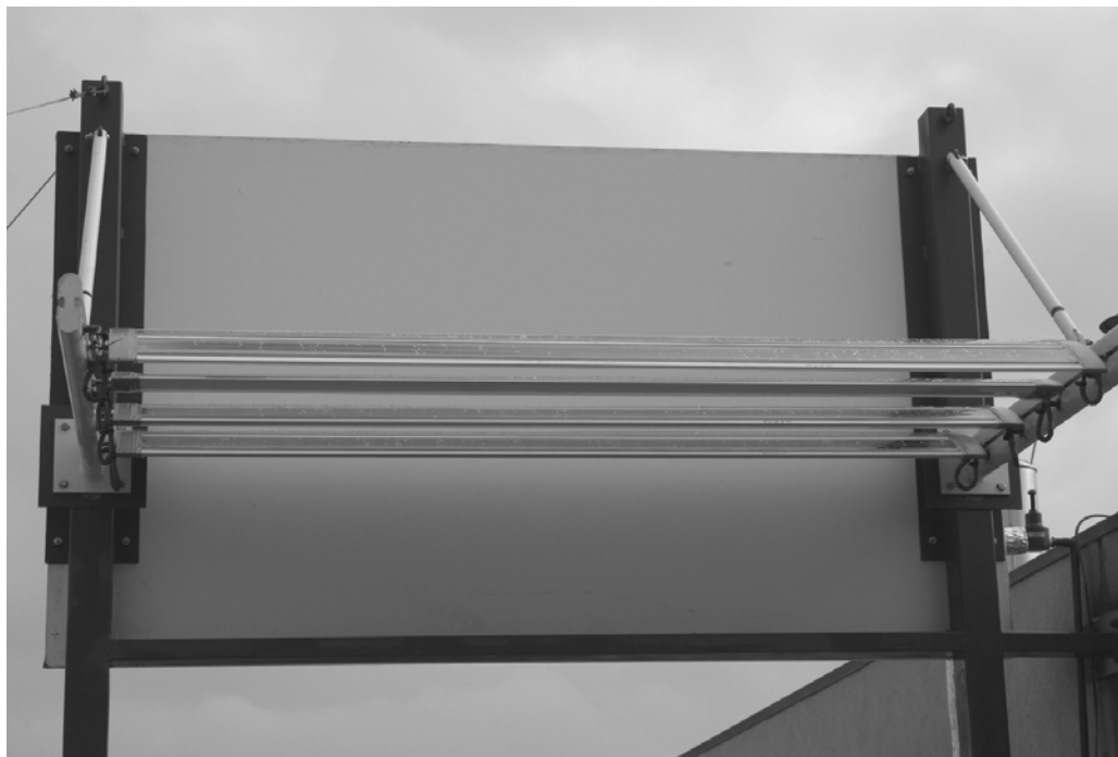
Fig.27 – View of solar louvre collectors.
