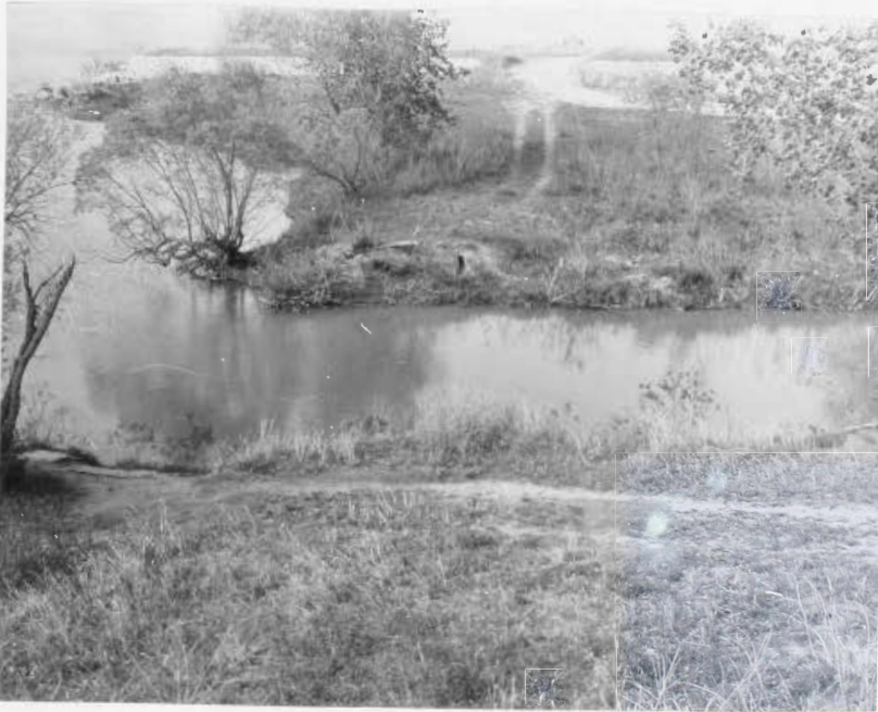
Figure 1. Gully in spillway at Antelope Lake, Graham County, Kansas.
