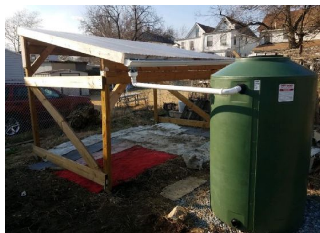
Figure 2: Rain catchment system, Fall 2018
