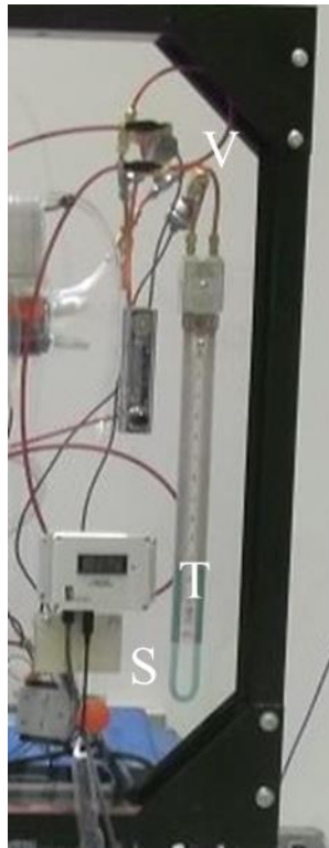
Figure 6. Oxygen-in-gas instrumentation on the control panel. Valves (V) divert the gas streams entering and exiting the membrane unit to the sensor (S). Mass percentage of oxygen in the gas stream is read on the transmitter (T).
