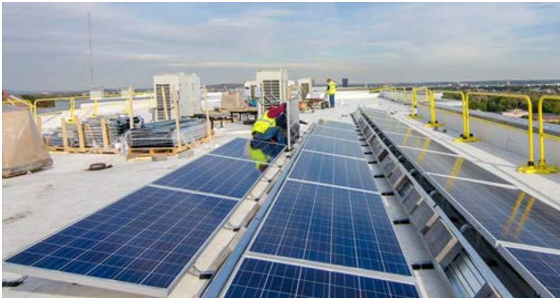
17 18 Figure 4. PV module on the rooftop of Celentano Hall 19
