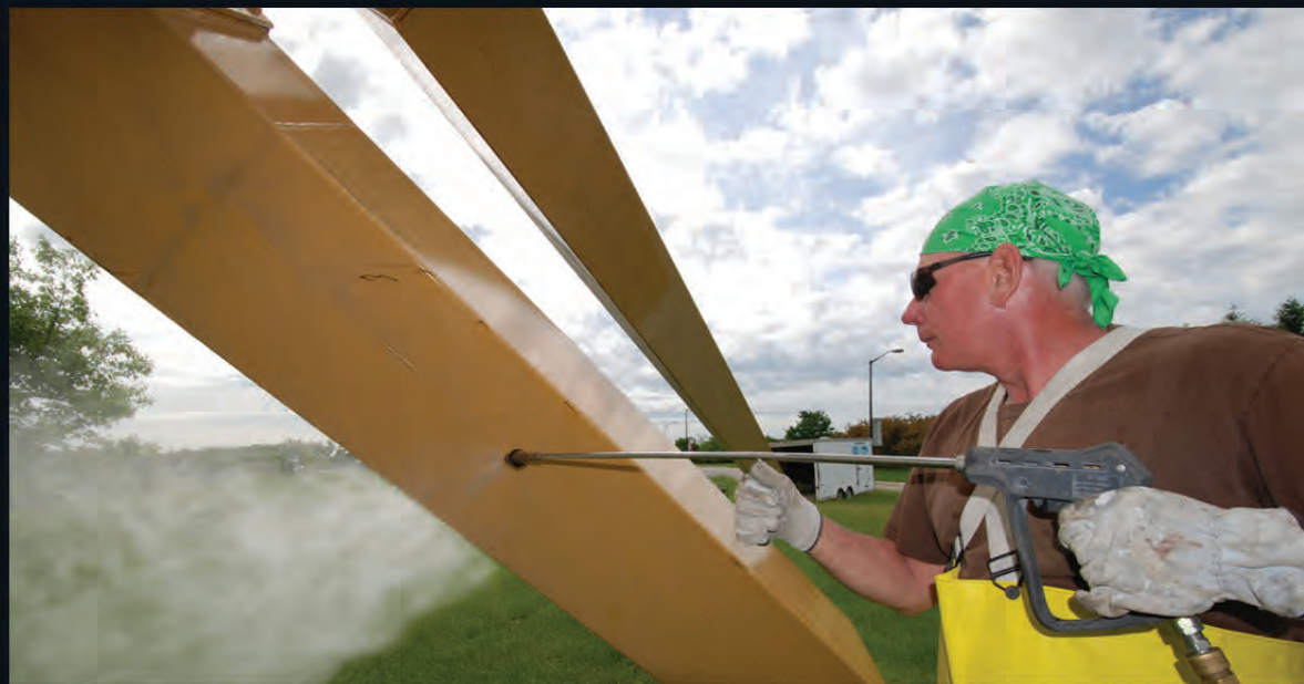
Above: Madison Coatings' Gary Goins conducted the work on Illinois Landscape No. 5 . Goins began by powerwashing the entire surface of the sculpture, removing the chalky residue of paint present since its last painting in 1997. Note the pale buttercream hue.
