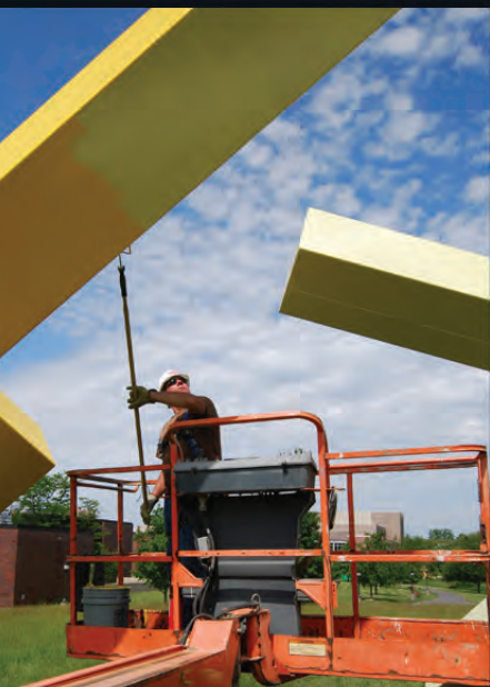
Above: Goins used an MBX grinder to remove rust from throughout the piece. He then "striped" and over-coated the entire artwork with rust resistant primer. He can be seen here applying the first coat of the Signal yellow hue chosen by the artist.
