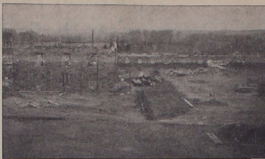
Shown above is an exterior view of the new dormitories for women students which are being erected in the area behind the college library. Work on the buildings was begun in June of the present year; the probable date of completion is September, 1957. (Photograph by S. P. Wagman)
