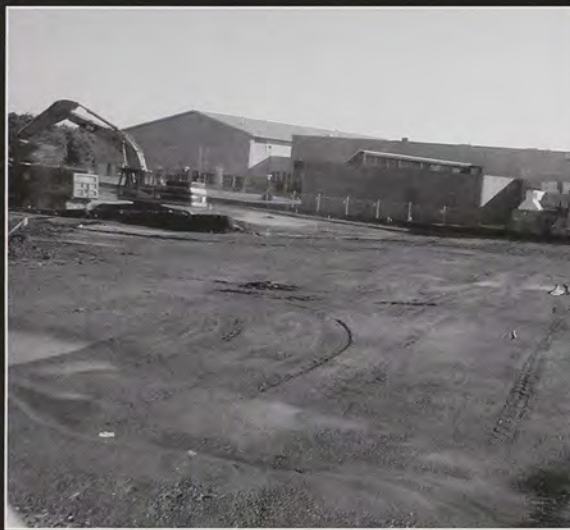
Above: Early work on the Performing Arts Center involved the clearing of some parking and grass with bulldozers and backhoes.
