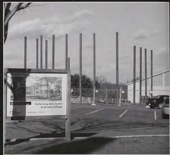
Above: Rising in the background of the artist's rendering of the PAC is the vertical supports for the structure.
