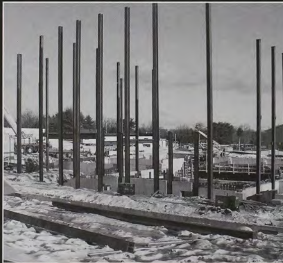
Above: Despite the snow, construction progressed on time with the vertical supports being added to the foundation of the building.
