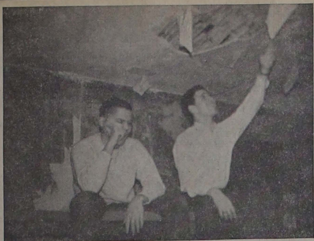
"Cheer up, Gary," Lew Linet counsels dormmate Gary Davis, as he pulls more plaster from the ceiling. "Maybe the Red Cross will send help into our little disaster area." No wonder Linet isn't too upset—his room was one of those which escaped the damaging effects of 724's burst water pipes last week.
