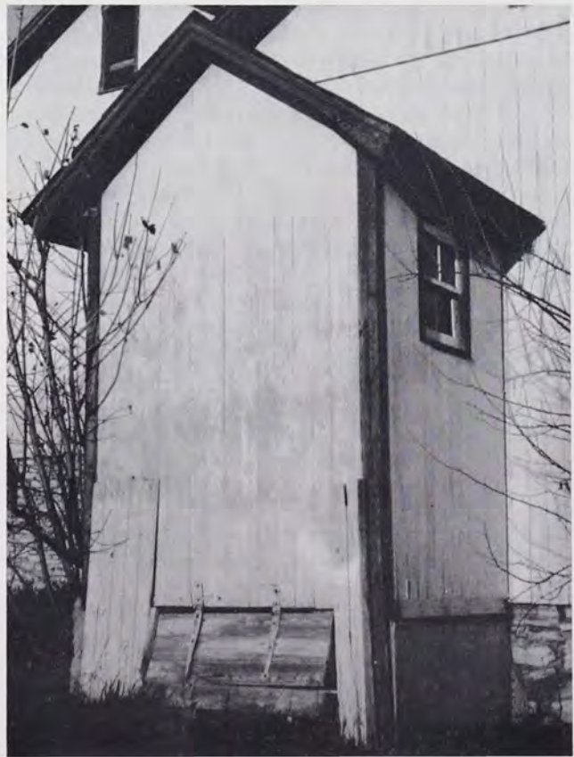
OUTDOOR PRIVY ATTACHED TO PIGSTY. Note hinged door for cleanout. Located on Henry Zug property east of Lebanon on Route 422. Dimensions: 6 ft. long, 5 ft. wide, 9½ ft. high (11½ ft. including roof). Pit: 3½ ft. long, 1½ ft. wide. Concrete foundation 2½ ft. high. Photographed 1962.
