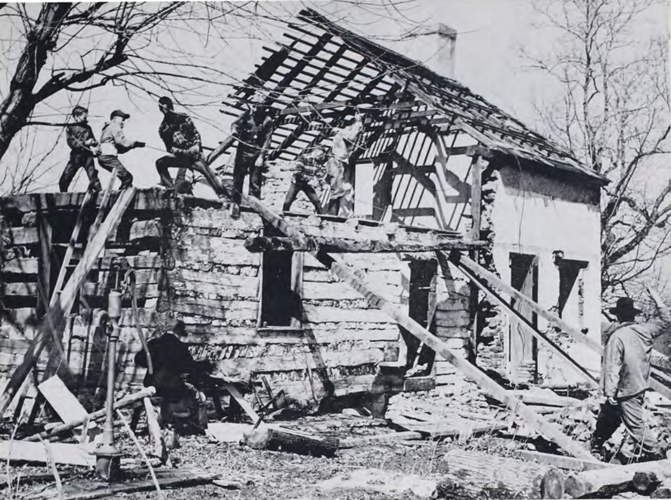
Dismantling the Johann Frey Swiss stone-and-log house, to be re-erected at the Goschenhoppen Open Air Museum. Living History Seminar boys assist under the direction of Clarence Kulp, Jr., right.
