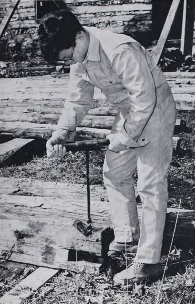
Logs are marked carefully for reconstruction on the new site. Living History boys participate under careful direction of trained archeologists and folk-architecture specialists.
