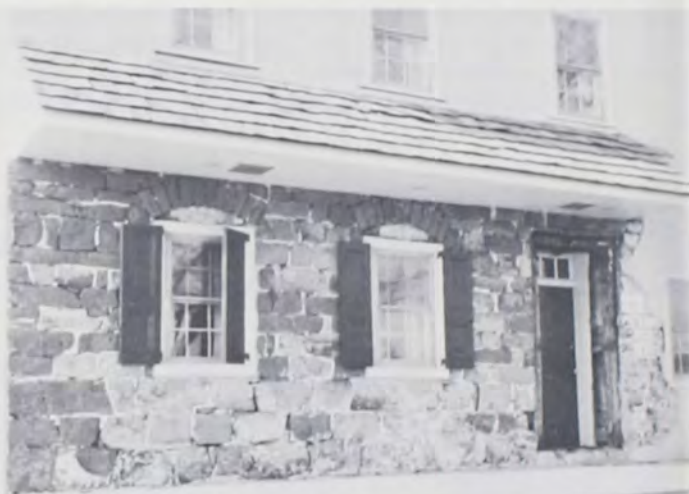
Front wall of Joseph Groof House, circa 1735, Valley of the Society Run, in process of restoration by Mr. and Mrs. John Philip Gebret, with technical advice and assistance by Goschenhoppen Historians restoration committee. The house is a Holland Dutch Mennonite town-house, built and arranged as a "Gemeinhaus" for dwelling as well as worship purposes. The original red tile roof will be replaced.
