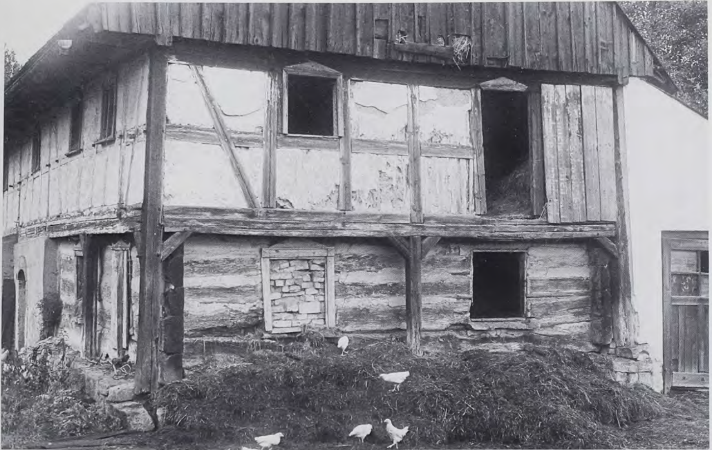
Fig. 12: False chinking on an Umgebände log and half-timber house in Zbylutów (Deutmannsdorf), a village in the Schwenkfelder source region in Lower Silesia, Poland (field research district 7). The split logs touch,
