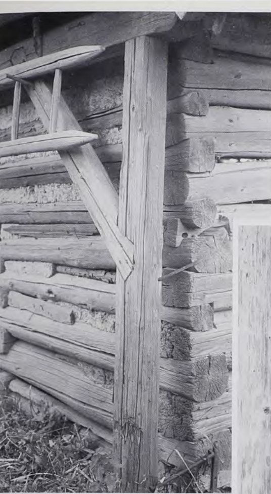
Fig. 14: Log barn in Horni Sloupnice (Obersloupnitz), near Litomyšl in the Loučná headwaters region of northeastern Bohemia (field research district 2). Note the two-sided hewing, thick timbers, and open chinks, some of which are filled with poles and daubing. Umgebinde construction is rare this far to the east.
