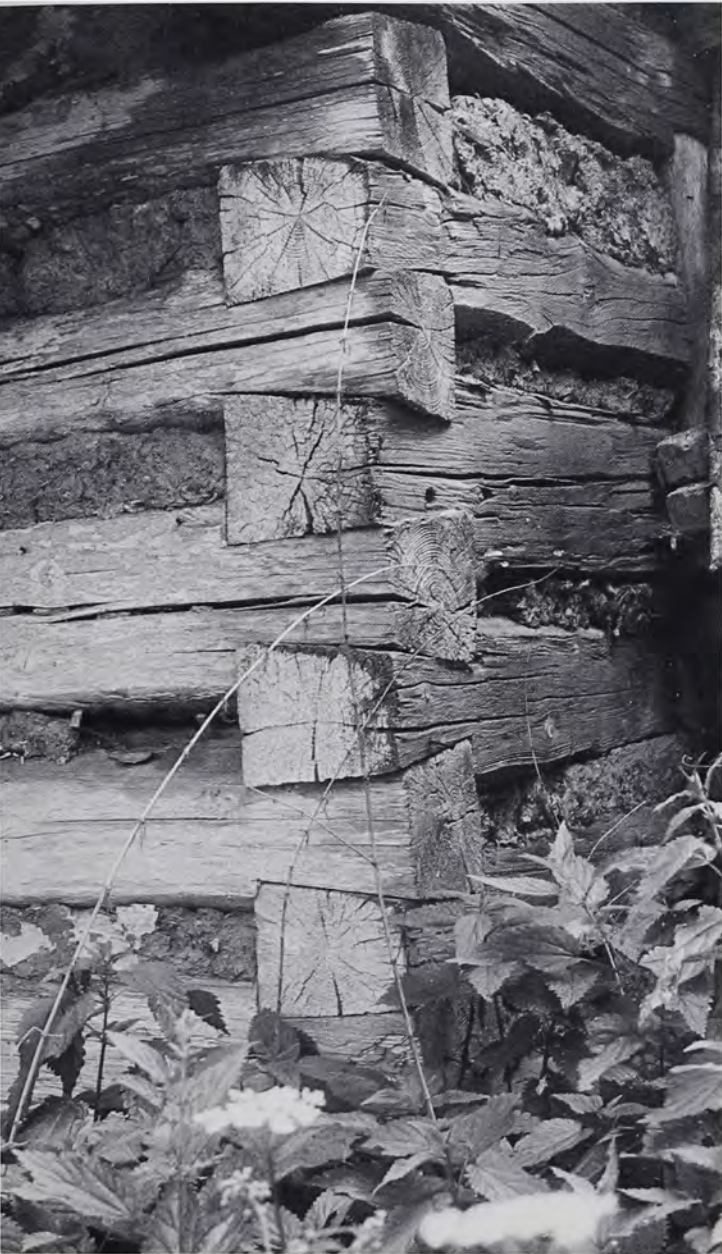
Fig. 6: Chinked log house in the Brethren source village of Kamenné Sedliště (Steinern Sedlitz), near Litomyšl in the Loučná headwaters region of northeastern Bohemia (field research district 2). Note, in the place where the chinking has fallen out, that the logs touch rather than being spaced apart. Note also the thickness of the logs, the two-sided hewing, the full-dovetailing, and the pegs to support the chinking.
