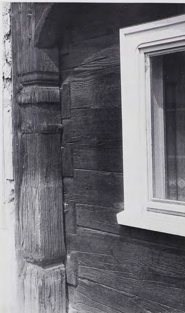
Fig. 11: Chinkless, hook-notched log house with Umgebinde construction, Hirschfelde, Upper Lausitz, German Democratic Republic (field research district 1).
