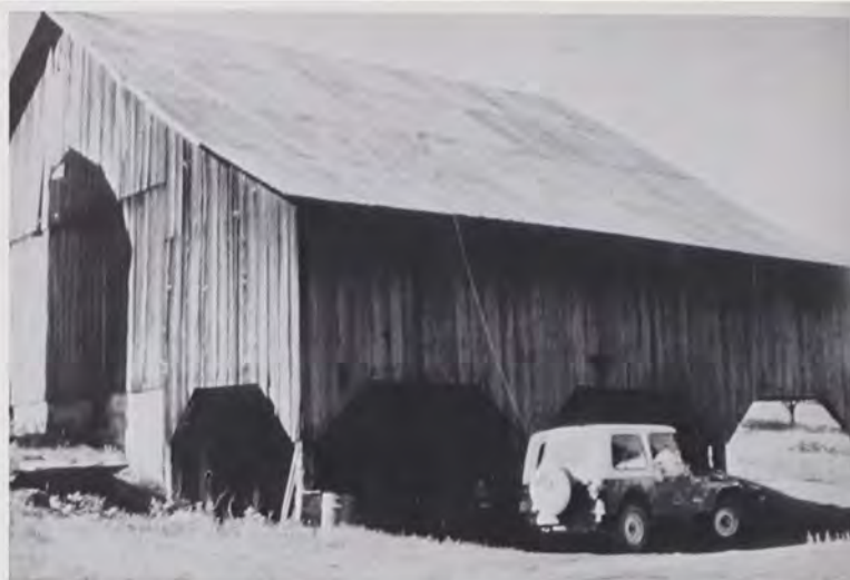
Nissel barn near St. Marys, Elk County, PA showing arched and supported forebay (c. 1880).
