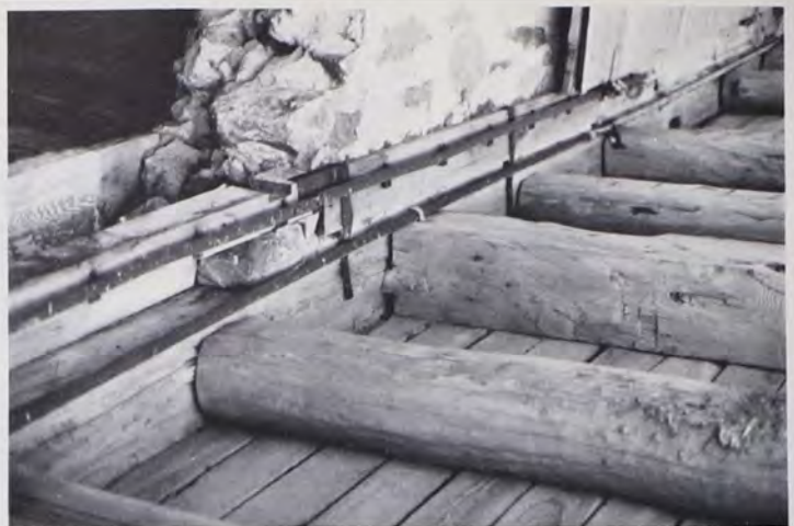
Rakow barn, Marathon County showing forebay joists mortised into stable wall sill.
