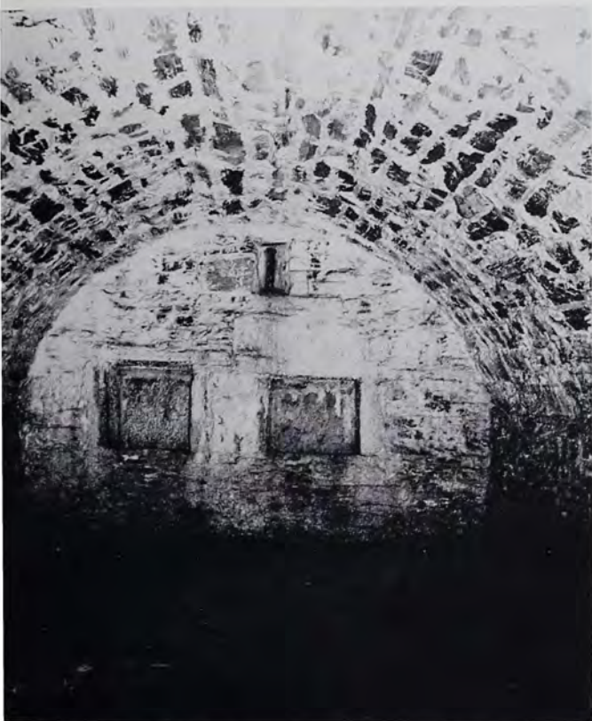
Cave-cellar, Keith-Moyer homestead, Schaefferstown. Interior, looking into the arch. Note the cooling closets and ventilating vent.
