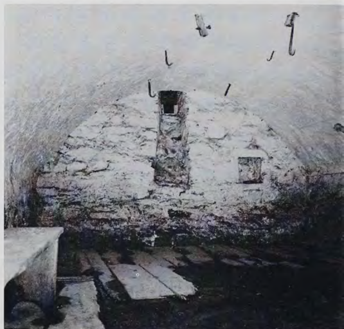
Arched cellar, Ulrich-Steimetz Farm, Lebanon County. Dimensions: approximately twenty-six feet long, thirteen feet wide, and seven and one-half feet high.
