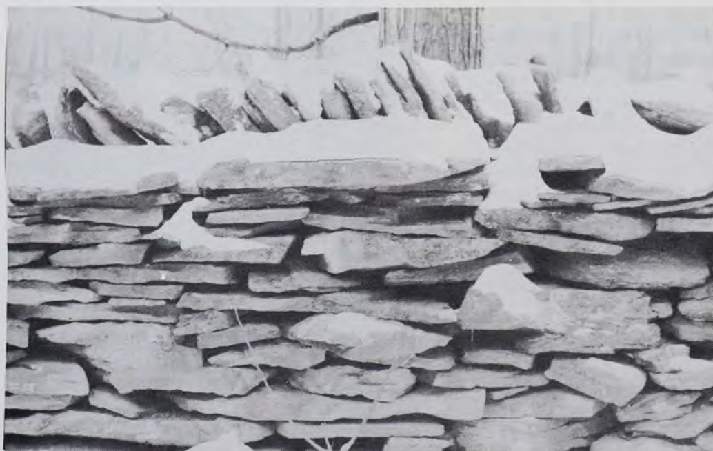
Stone wall near Hop Bottom with a vertical stone cap. This finish helped to stabilize the wall.
