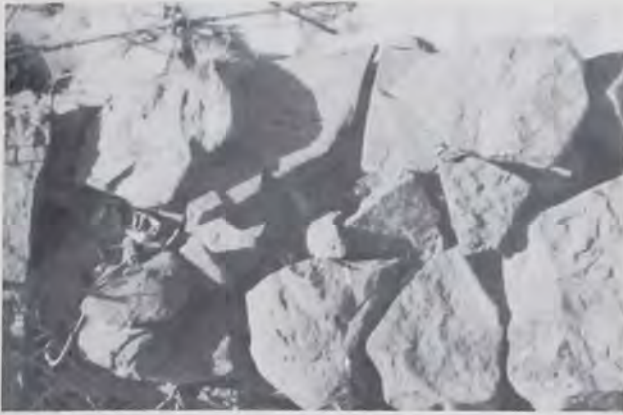
Top of a stone wall near Springville showing the two parallel faces and the rubble fill placed between them.
