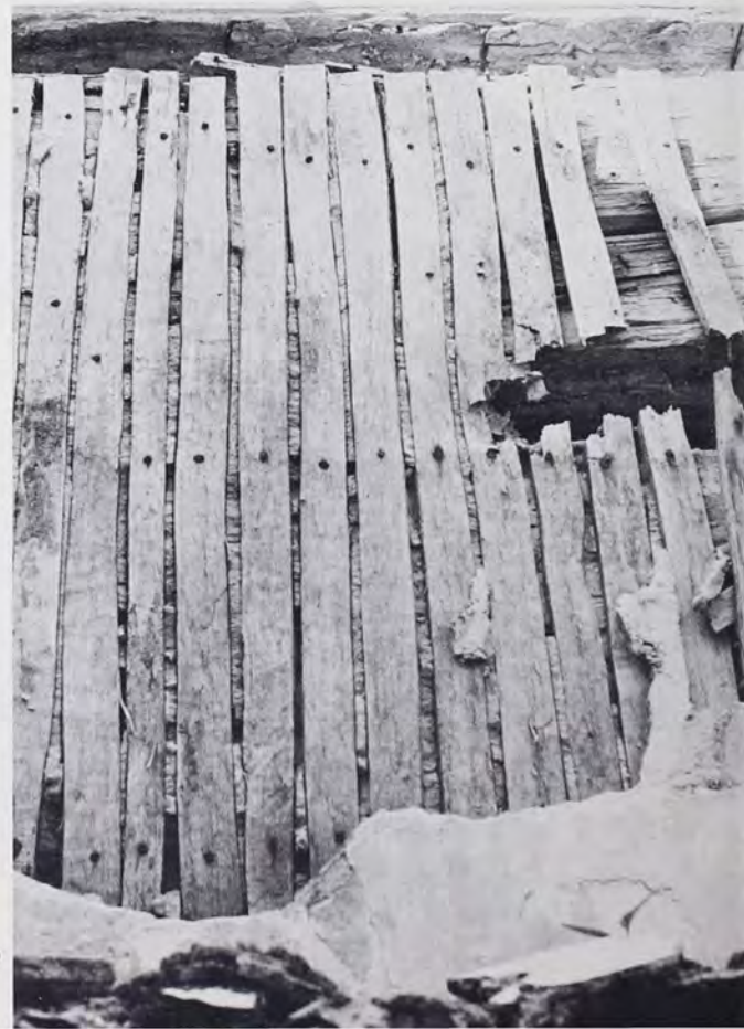
Vertical Lath. Lath of the second story walls seen through a hole in the kitchen ceiling.
