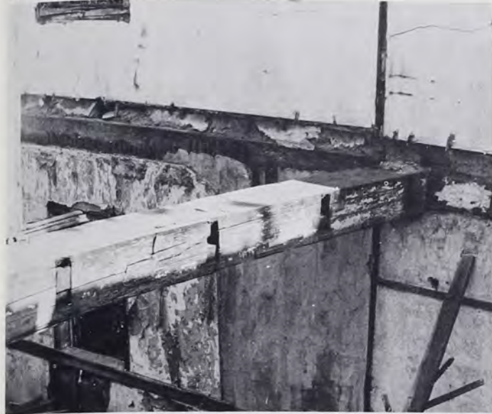
Summer Beam. Summer beam seen from the second floor. Note the notches for the joists, the vertical lath, and the groove in the plaster which marks the partition that bisected the room behind the chimney.
