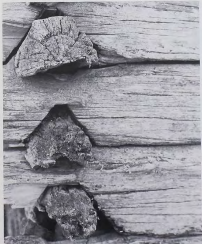
Fig. 11: Blunt-apex V notching, mixed with undersided saddle notching, on an outbuilding in a still-occupied Finnish farmstead near Rödjäfors, Värmland province, Sweden, in the Finnskog high ground very near the Norwegian border. Removal or deterioration of crowning on three logs reveals the notch structure. (Photo by T.G.J., 1985.)
