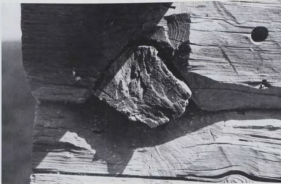
Fig. 9: Hewn, blunt-apex V notching from the sixteenth century at Vang, Hedmark province, Norway, and now in Hedmarksmuseet og Domkirkeodden at Hamar. On the log with butt end toward the camera, the crown and
