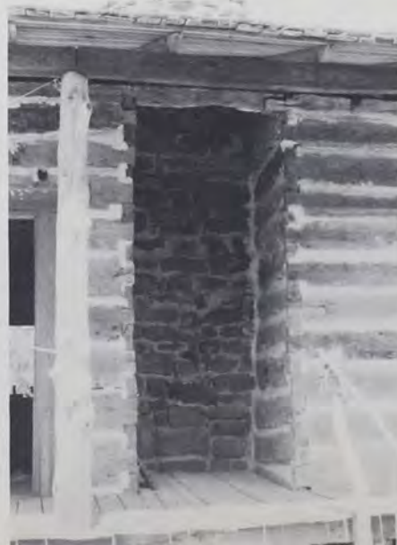
Fig. 4: Unused space in front of the chimney, Knowles-Townsend house, Gonzales, Tex. See also Figs. 1 and 2H. (Photo by T.G.J., 1989)
