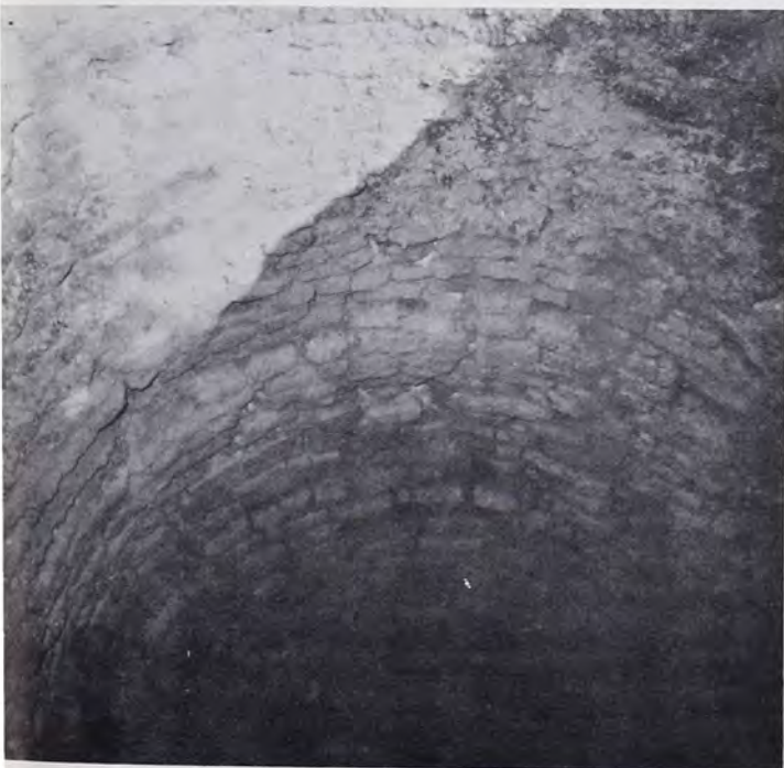
Looking down into interior of Schoener limekiln shaft. Open shafts like this one are difficult to find because most of them have been filled in. Photo taken 1962.
