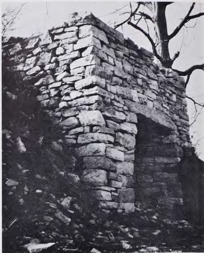
Side view of limekiln showing how kilns were built into steep hillsides. Shafts were filled on the upper level and the burned limestone removed from the lower level. Ray S. Walters, aged 74, Buffalo Springs, who helped operate the kiln during earlier years, at right (1963).
