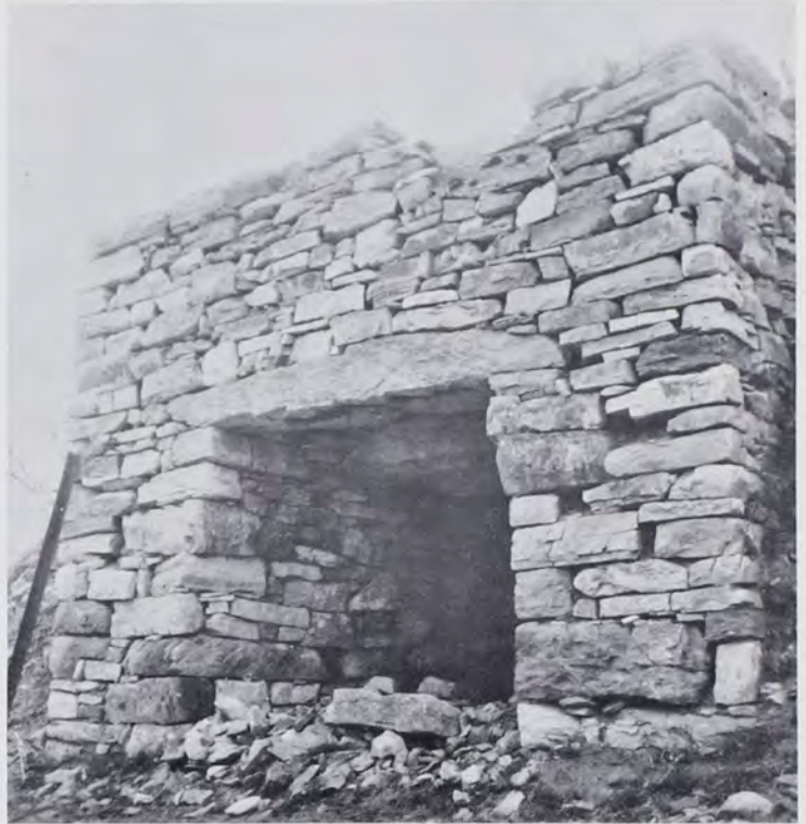
Flat corbelled arch in limekiln located in Buffalo Springs, Lebanon County, Pennsylvania, on Ammon Binner Farm (1963).
