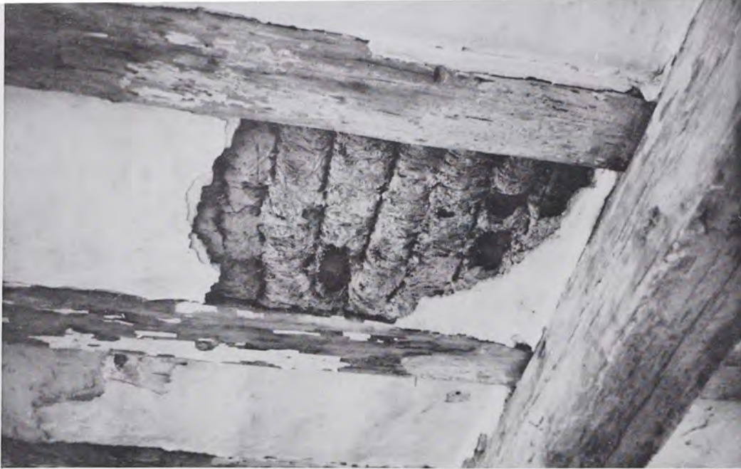
Plate 9 Ceiling of the Herr House with view of the hand-hewn joists and slats wrapped with straw and mud. These are fastened between the joists and then covered over with plaster.
