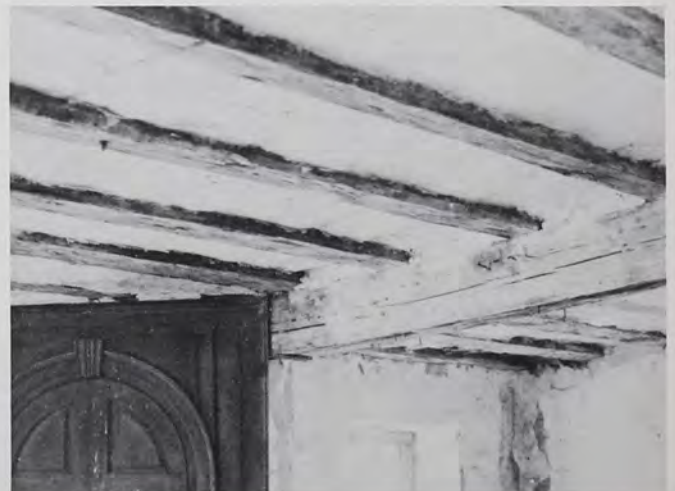
Plate 10 Another view of the ceiling in the main room of the Herr House. Lime plaster covers the slats between the joists and is almost flush with the joists. The top of a large cabinet can be seen to the left.
