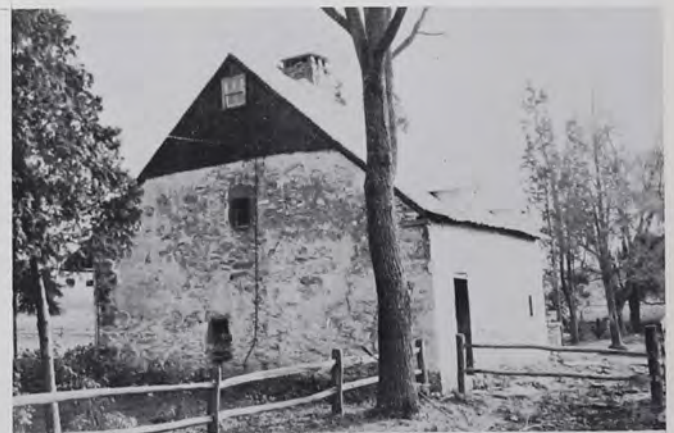
Plate 18 A view of the rear of the Zeller House and its north gable. The window at the center, near the ground, opens into the kitchen. Like the one above it, it too is stone-framed.
