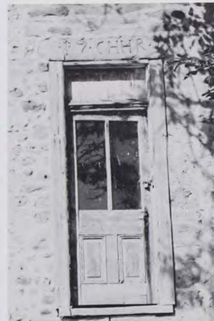
Plate 6 The front door of the Herr House is shown here with wooden frame and inscription over the door.
