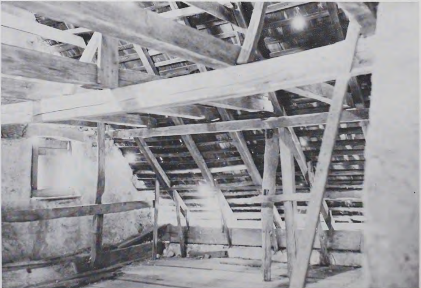
Plate 26 A view of the second level of the Herr House showing the roof construction (framing) and the alterations made to cure tobacco. The summer beam runs directly across the photograph.
