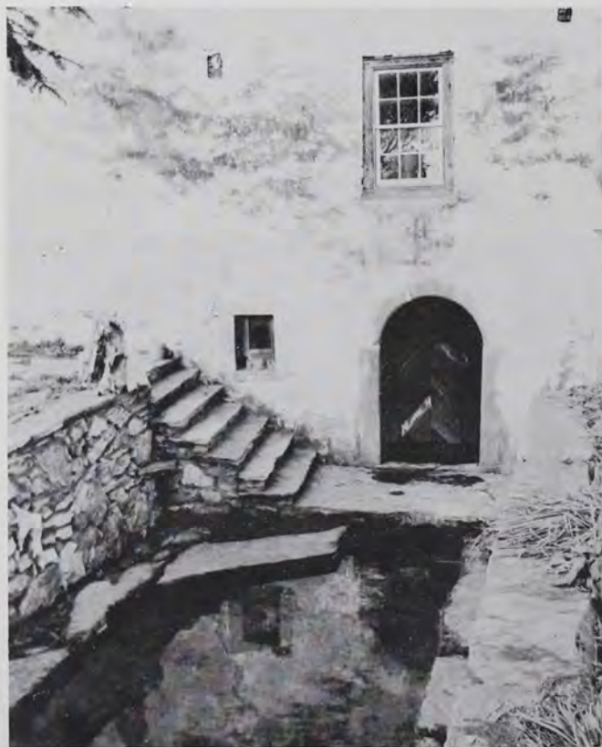
Plate 24 This view shows the diagonal board door that leads into the spring room of the Zeller House. It is framed in dressed limestone.
