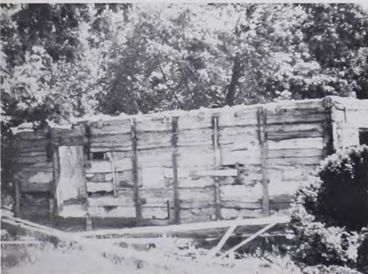
Turnpike House-West side. The plaster patch just right of center is the Seelenfenster. Note the disturbance in the framing of the window.
