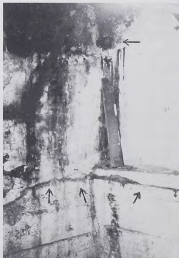
Right-hand corner of fireplace in the Adams County log house. Top arrow indicates position of the iron ring which supported a wooden crane. The lower arrows indicate the two foot high ledge running along the back wall and the right jamb.
