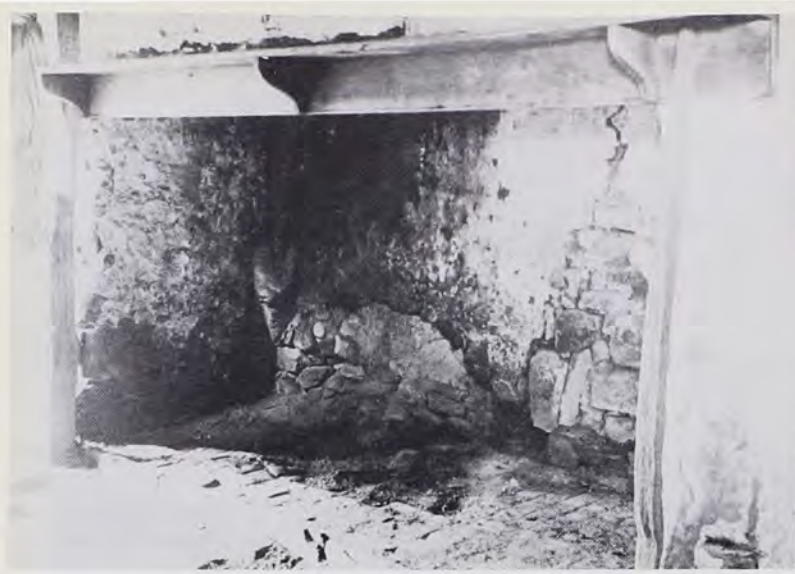
This ca. 1925 photograph of the kitchen fireplace in the Herr House shows a clear disturbance of the mortar on the left jamb and back wall near the fire crane, an area that would have been occupied by a raised hearth. The missing mortar to the right marks the original heating-stove opening.
