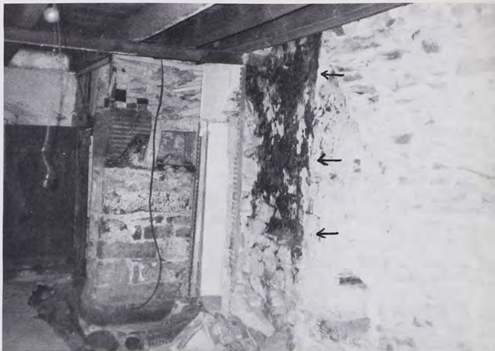
Kitchen fireplace in the ca. 1735 Antes House. The arrows indicate the smoke channel; note the relationship of the smoke channel to the stove opening.
