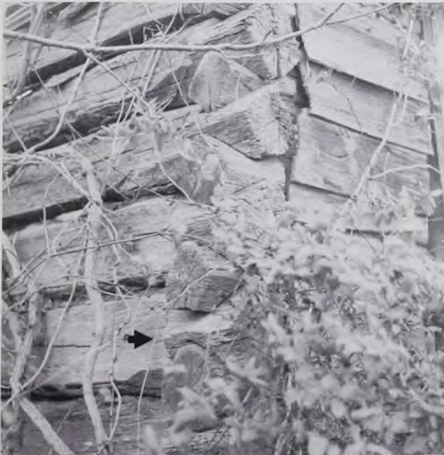
Fig. 7: The arrow indicates where the outer ridge of the diamond projection extends beyond the hewn wall surface in an awkward manner; Franklin County, North Carolina. It represents type F on Fig. 10. (Photo: T.G.J., 1983.)
