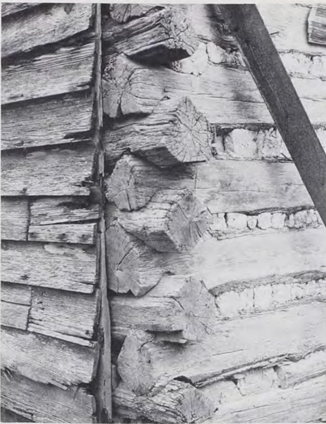
Fig. 8: The projecting ridge of the diamond notch has been planed away where necessary on this Franklin County, North Carolina, structure. (Photo: T.G.J., 1983.)
