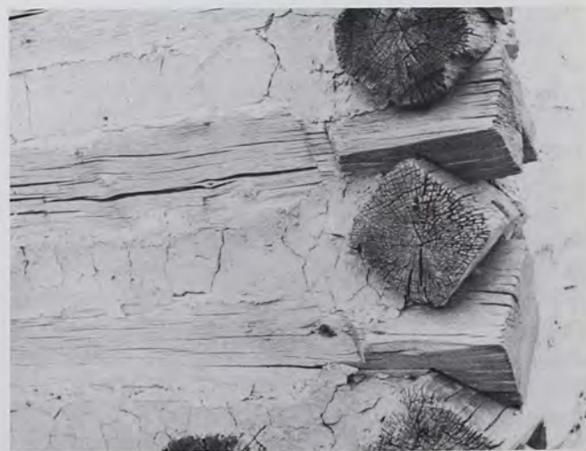
Fig. 5: Hewn diamond notching; Fort Gaddis, Fayette County, Pennsylvania, circa 1765. It represents type F on Fig. 10. (Photo: courtesy Western Pennsylvania Architectural Survey, Carnegie Library of Pittsburgh, item no. F1-107d.)
