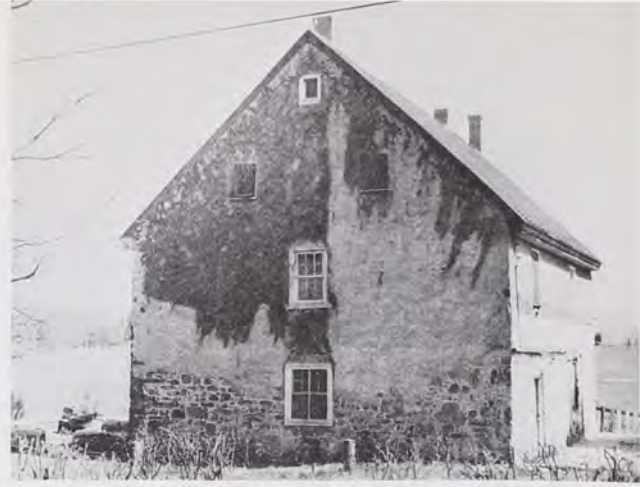
The north gable wall of the Antes House. Note the double attic indicated by the two levels of smaller windows above the second floor.
