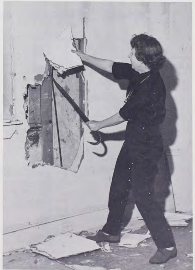
Off comes the plasterboard on wall of 1696 brick section of Thomas Massey House, with Clarissa Smith (co-author) wielding the crowbar.
