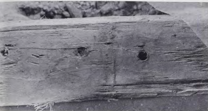
Original floor joist in 1696 section of Thomas Massey House, showing peg holes and built-up dirt marking joint between the floor boards.
