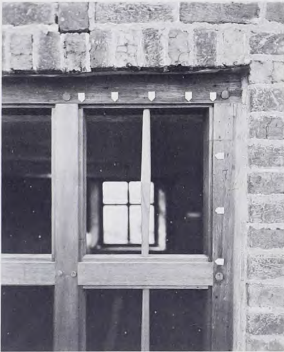
Original 1696 casement window frame (north side) showing nail holes and restored center members. Arrows indicate glass size, 4" x 6".
