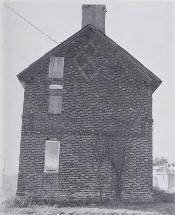
Gable end (east side) of Thomas Massey House in 1963. Brick section was built in 1696; two later stone additions 1730, 1840-1860. Note pattering in brick, found in early English houses of the Delaware Valley.
