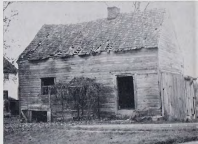
The Pott Cabin—Oley Valley. Built over a spring with running water in the cellar. Original casement windows.
