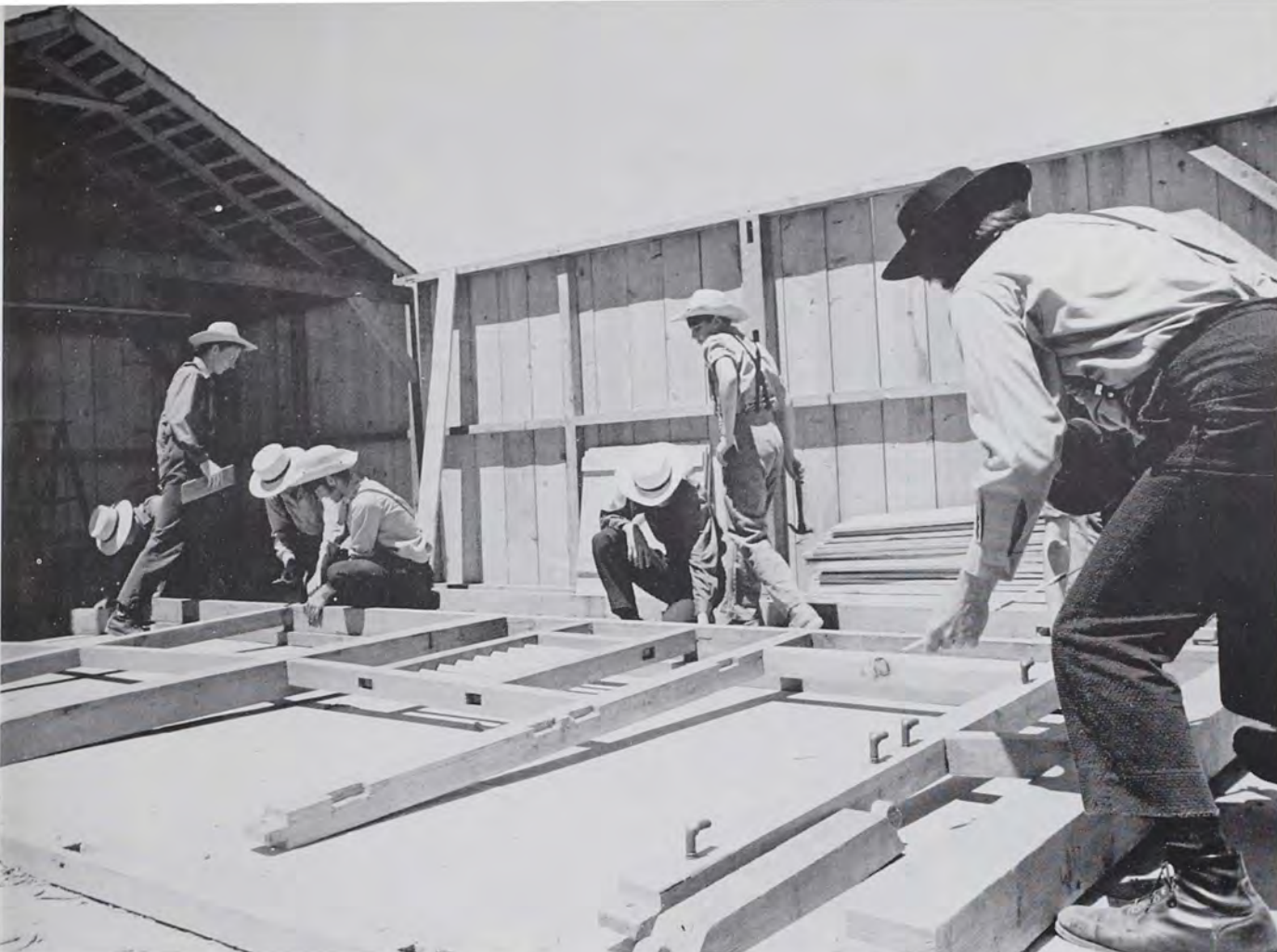
At the 1971 Kutztown Folk Festival a section of wall between two bents is being assembled. The top of the wall is laid toward the center of the barn and the bottom of the wall toward the outside. Notice how the uprights are tongued so that they fit into the grooves in the beam along the foundation. In each tongue is a hole for a wooden peg and through each groove is the corresponding hole. On the picture from left to right are Gary Schukraft, Kane Scheidt, Peter Lilienthal, Joseph Tengel, Richard Gougler, Jr., David Roth, Gary Bond and Lester Lutz, all from Berks County.
