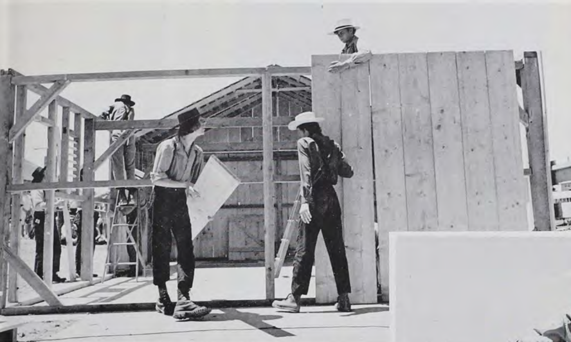
Now that the main structure is standing, the men are putting on the siding. Since the structure was put up 16 times during the festival, the siding was not nailed fast as is usually done. The man in the center is carrying a board at the top of which can be seen the hooks which he will place on the nails that can be seen along the top beam. In the foreground are Williams, Gougler and Lilienthal.
