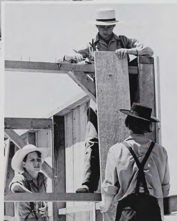
This is a closer view of fastening the sides. If one looks closely at the brace behind the boy with the hammer, the wooden pegs can easily be seen at each vertex of the triangle. With careful inspection, two of these can be seen on the brace in the foreground. The ends of the pegs have already been sawed off. Shown are Roth, Lilienthal and Williams.
