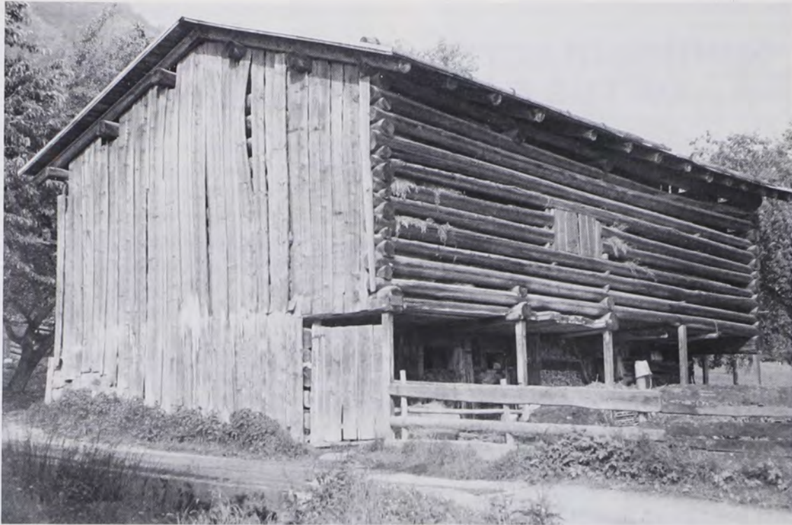
Fig. 2: Double-crib log forebay barn in Saas, Prätigau. Note the wooden forebay support posts; the window in the forebay, to illuminate the threshing floor and to
