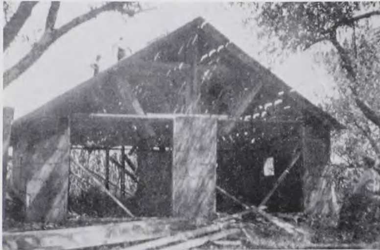
As at all Junior Republics, carpentry training was provided for the male citizens. Here the boys of the GJR of Western Pa. erect a new machinery house. Citizens cast the block, did the wood work, and erected the walls without adult supervision (ca. 1927).
