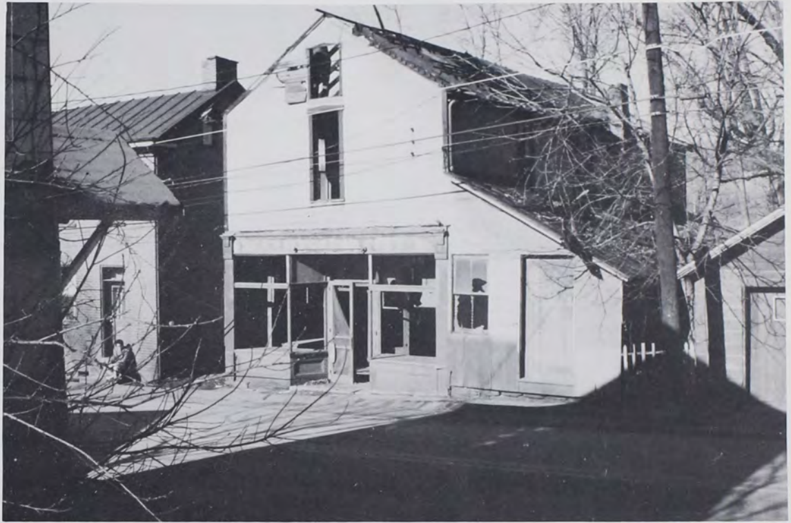
Store being demolished in 1990; note the two display windows on either side of the door. A shed roof extended over the sidewalk.
