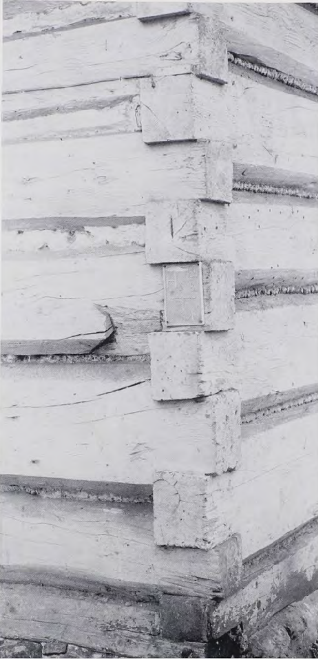
Fig. 17: Chinked, square-notched building in the town of Zakopane, Galicia province, Poland. Square notching is common in this Slavic area. (Photo by T.G.J., 1982)
