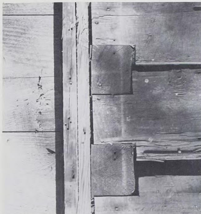
Fig. 8: Square notching on sawn logs, Fanthorp Inn, at the town of Anderson, Grimes County, Texas. The inn, built in 1834, was covered with siding at the time of construction. (Photo by John Weaver, 1985, and used by permission of the Texas Parks and Wildlife Department, Austin.)
