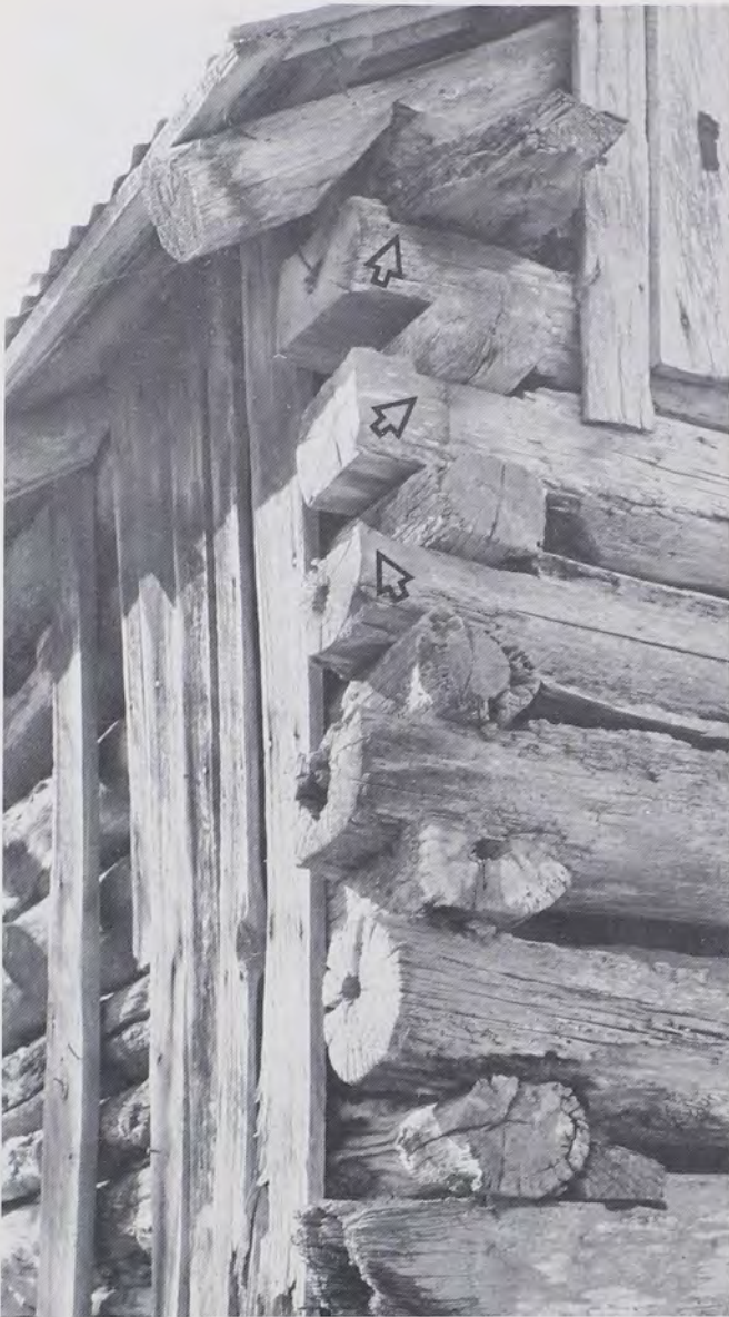
Fig. 25: This highly significant structure, a barn standing alongside highway 76 at its junction with road VV in Taney County, Missouri Ozarks, displays throughout a mixture of crowned vertical double notching (arrows) and square notching. It further combines round-log, hewn-log, and hewn-only-near-the-corners shaping. Locationally, it represents a giant stride eastward from the Mountain West towards the Pennsylvania hearth of Midland carpentry, in a purely upland southern cultural context. It, together with a sprinkling of similar Midland structures in the East, convinces us that all of these are archaic features belonging in the Pennsylvania log carpentry tradition. (Photo by J.T.K., 1989)
