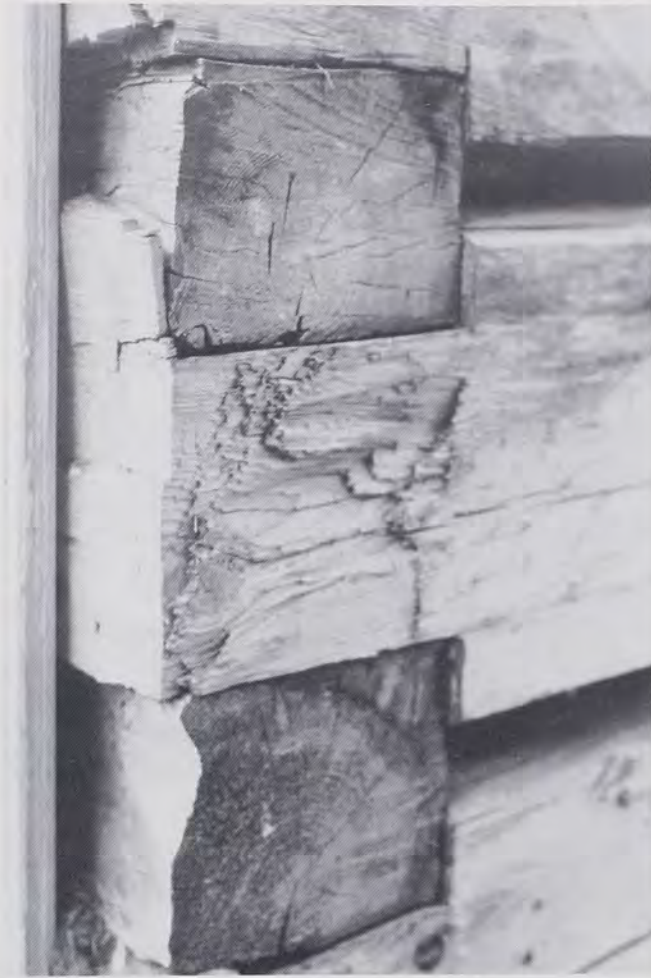
Fig. 21: An obvious instance of vertical double notching sawed off to form square notching, here done so ineptly that abundant evidence of the alteration survives. The building, from the Swedish city of Östersund in Jämtland province, now stands in the Jamtli open-air museum in the suburbs of that city. (Photo by T.G.J., 1985)
