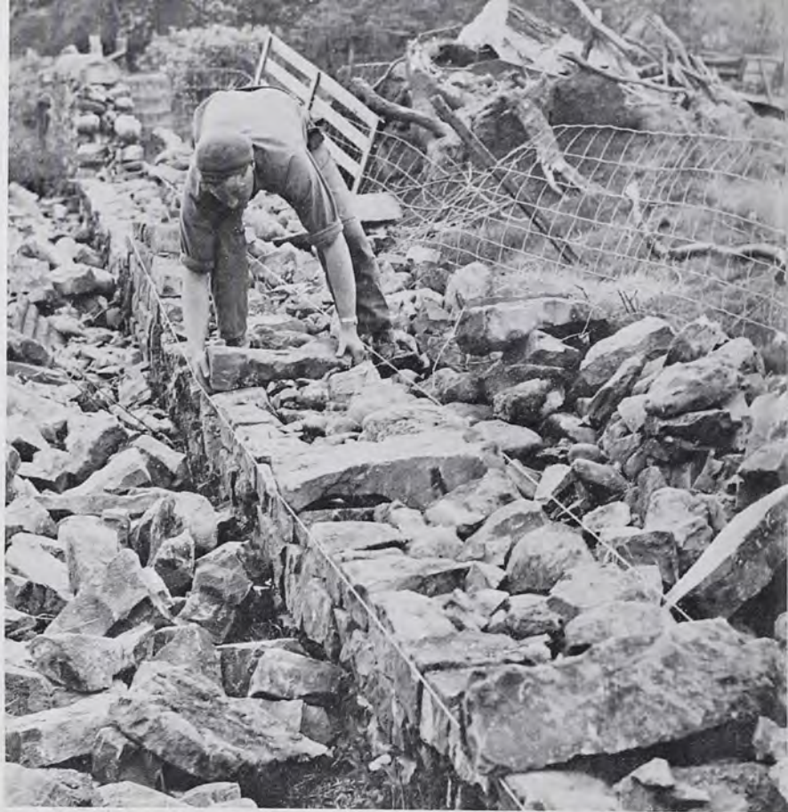
Drystone walling. Ribblesdale, Yorkshire. Laying "throughs" across from side to side of the wall about 2 ft. from the ground to bind the two faces together. The large section being repaired is built up from stones from the collapsed section and a line is used as a guide in setting each "course" just a little behind the one below to guide the wall correct "batter".
