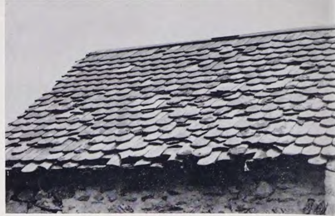
"Staggered" tile roof on bake-house, Troutman farm, north of Womelsdorf. Note the half-tiles.
