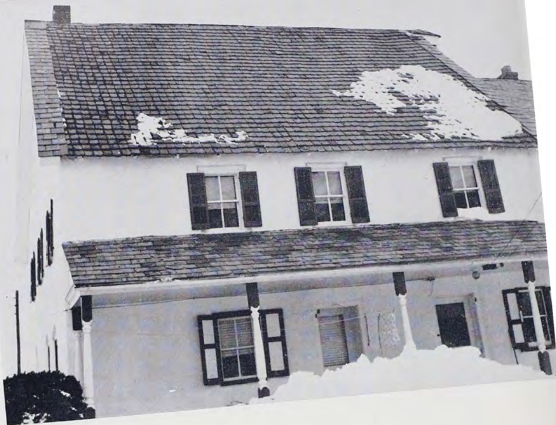
Original tile roof (south side only) on the Isaac Long House, Landis Valley, Lancaster County, built circa 1760. Tile laid with vertical and horizontal joints.
