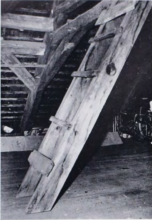
Wooden ladder with 1" opening at bottom and 3" opening in center, believed to be a key part of grain hoist.
