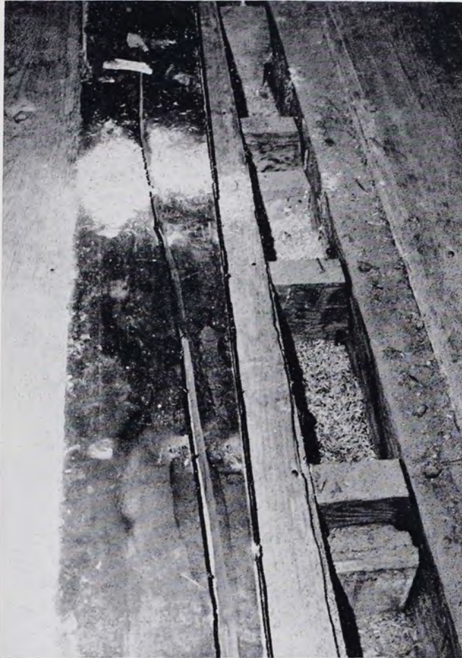
One attic floor board has been removed showing grain between attic floor joists of Mock house.
