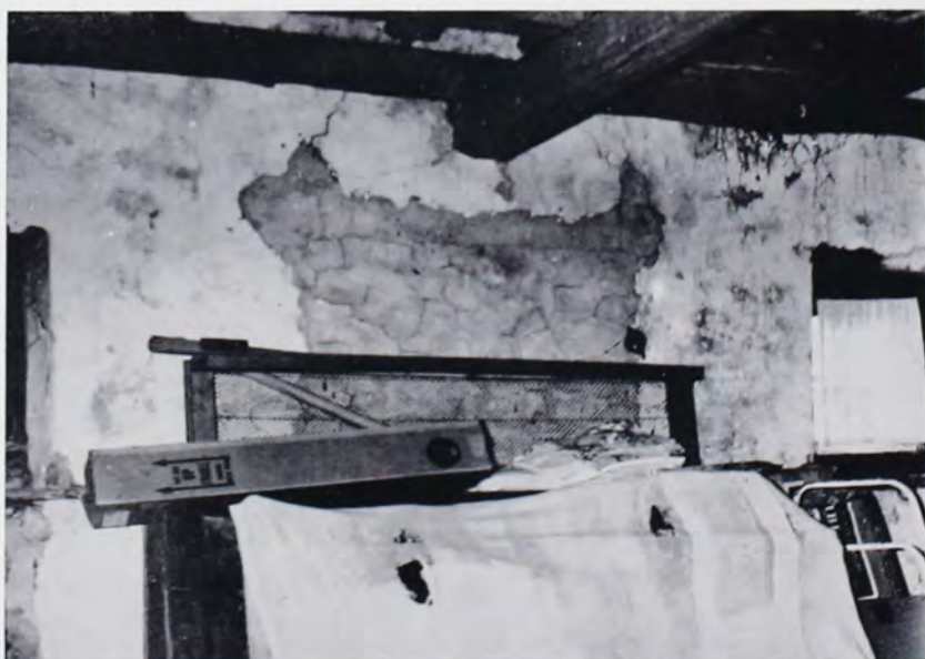
New mortar on inside wall of west gable of Viehman house marks area once open for hoisting grain to attic.
