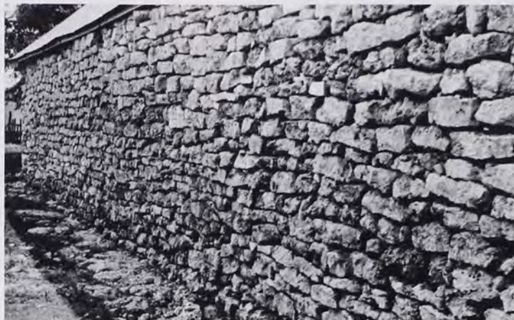
Figure 10: Stone wall on the north side of the Hamic barn. The "mountain mud" mortar has weathered out, leaving essentially a dry rock wall. Photo 1979 by the author.
