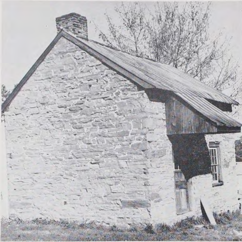
The hard, crisp lines of the limestone and mortar form an interesting pattern on the west wall of the doctor's office. The tapering width of the trim under the roof indicates its early age and remarkable preservation.
