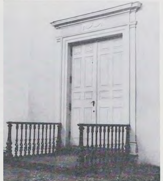
The brick walk and iron balusters provide an interesting approach for the simply executed doorways.
