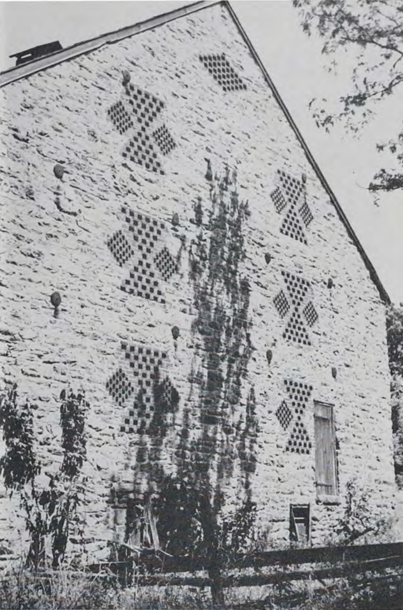
This is a close-up view of the inserted brickwork designs in the stone-end Gorsuch barn.
