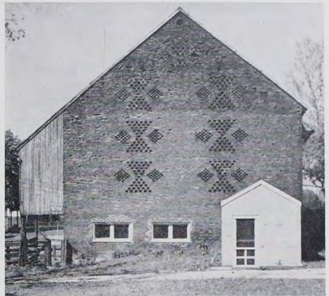
"SOFT BRICK" —Of the many brick-end barns examined by the writer, this is the only one that suffered severe damage to the wall face. Note, however, that it is the soft brick used that was at fault here, not the skill of the bricklayers who fashioned the designs. The owner says that many birds peck at the soft brick to sharpen their bills. This, together with the effect of the weather on this poor-quality brick, has badly marred the beauty of the wall.
