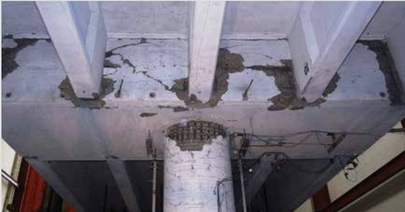
Spalling around dowel bars in girder connection region
