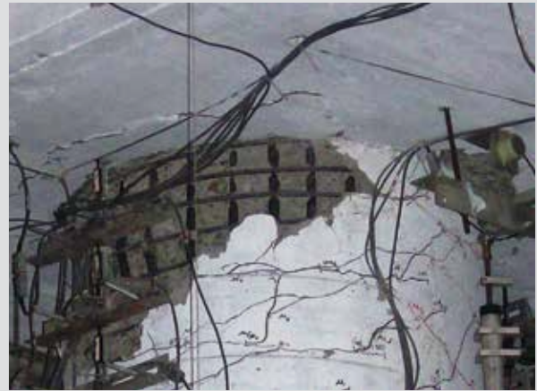
Buckled bars in the column top plastic hinge region
