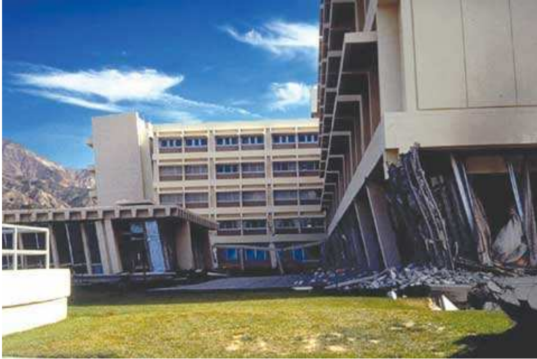
Figure 1.2. Seismic damage to Olive View Hospital, 1971 (USGS, 2005)
