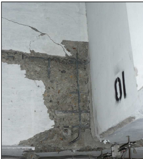
b. Deterioration of as-built connection
