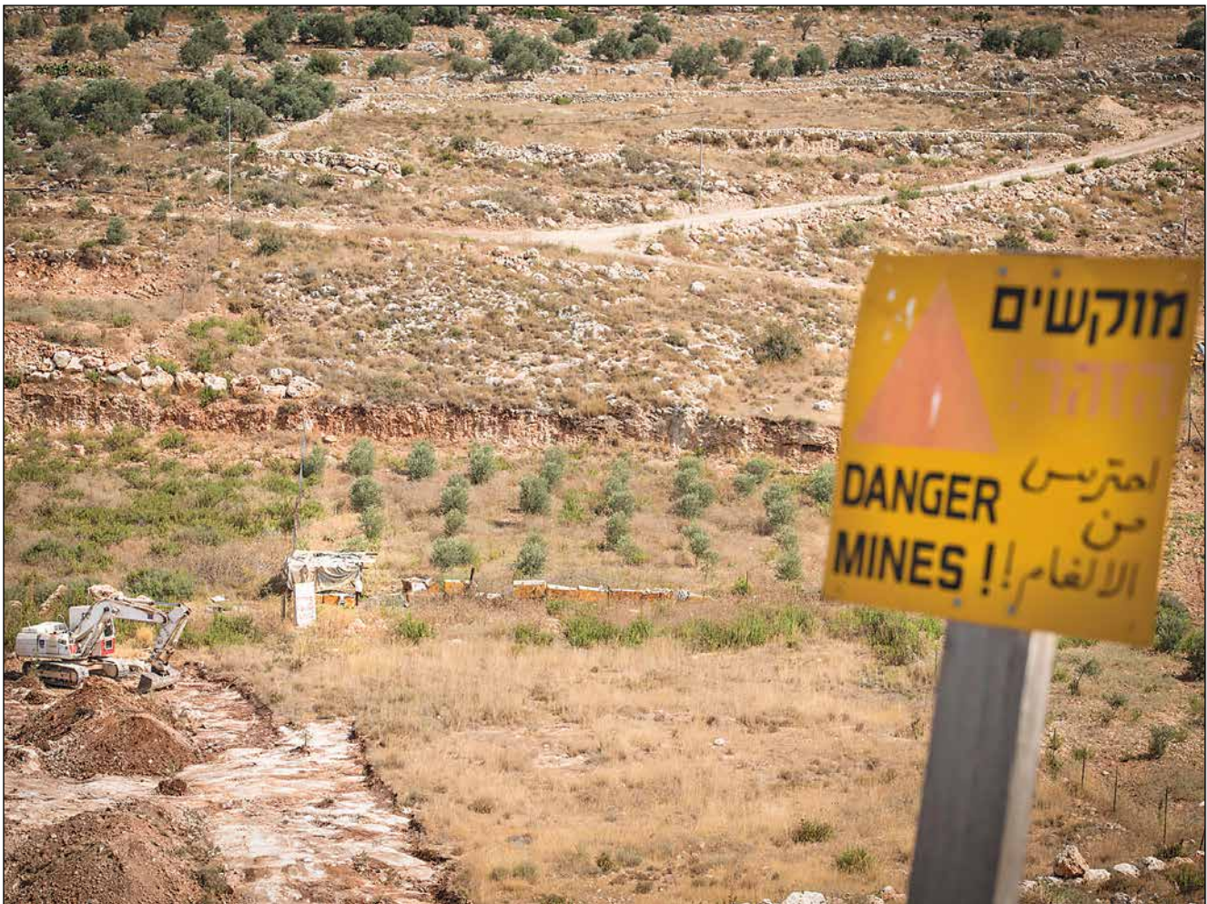
Using heavy equipment on a clearance task funded by PM/WRA, HALO demines in the West Bank. Photo courtesy of HALO.
