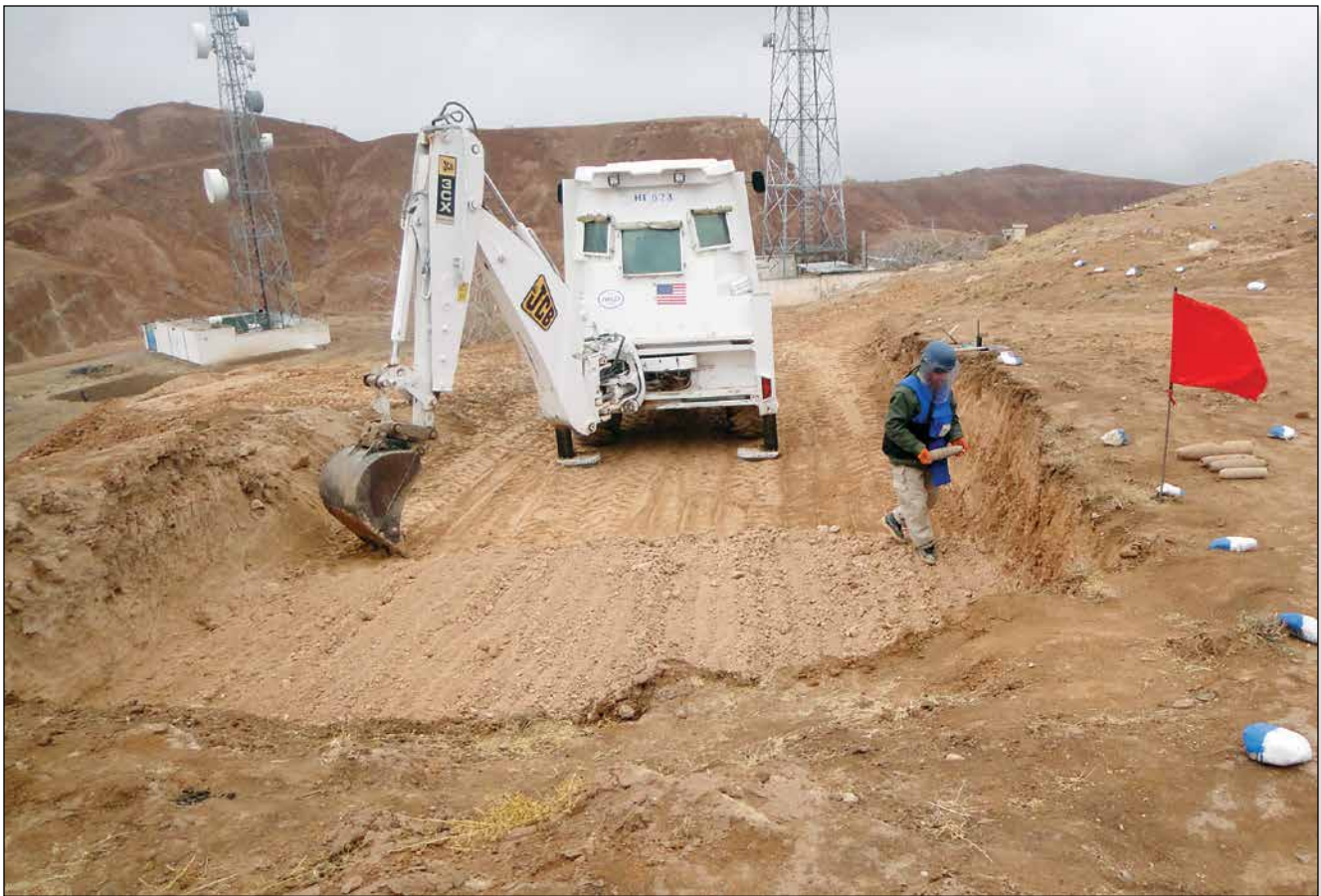
With PM/WRA funding, HALO conducts mechanical clearance near communication towers in Samangan Province, Afghanistan. Photo courtesy of HALO.
