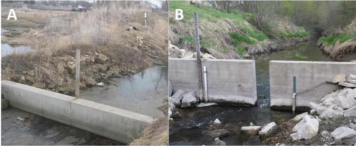
Figure 1.21. County Ditch 57 diversionary weir (A) and rate control weir (B). The diversionary in this watershed is designed to slow discharge and allow sediment to settle on the channel bottom. It also diverts water into a surge pond for further treatment. The rate control weir is designed to reduce the amount of water leaving the watershed and also to slow discharge upstream to allow sediment to settle on the channel bottom.
