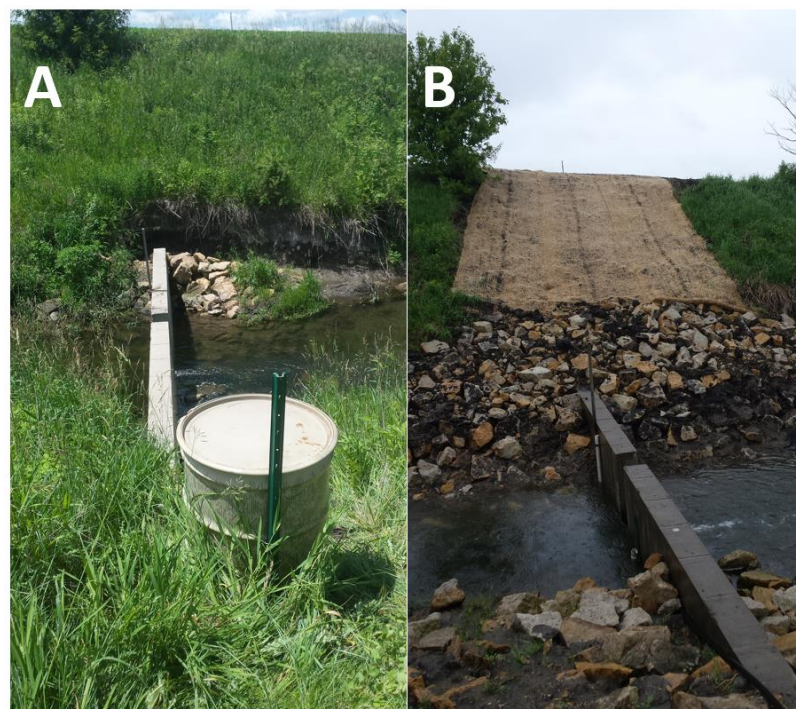
Figure 2.9. Pictures showing bank failure and repairs at CD001. The left image is from June 2015, while the right image is from May 2016.
