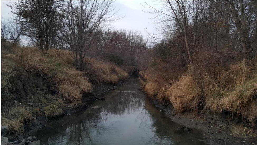
Figure 2.10. Picture showing bank failure on both sides of the channel, immediately downstream of CD001. A slump can be seen circled on the left side of the image, while the right bank has experienced undercutting and is susceptible to slumping.
