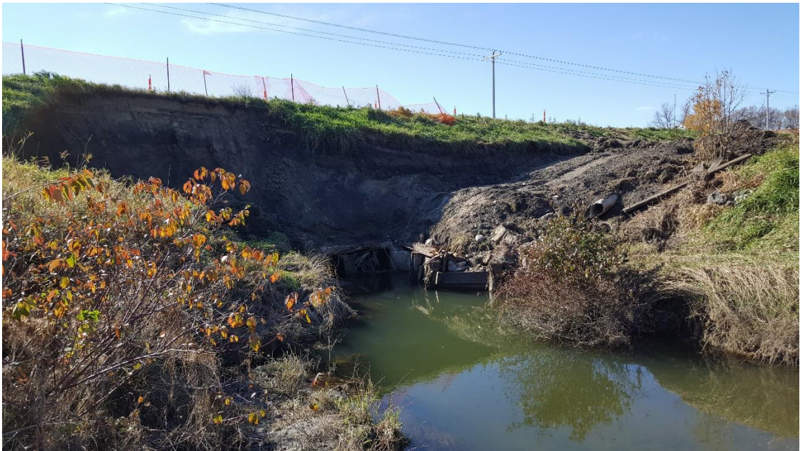
Figure 2.11. Picture (October 2016) showing failure of the box culvert under County Road 4, immediately upstream of CD001.
