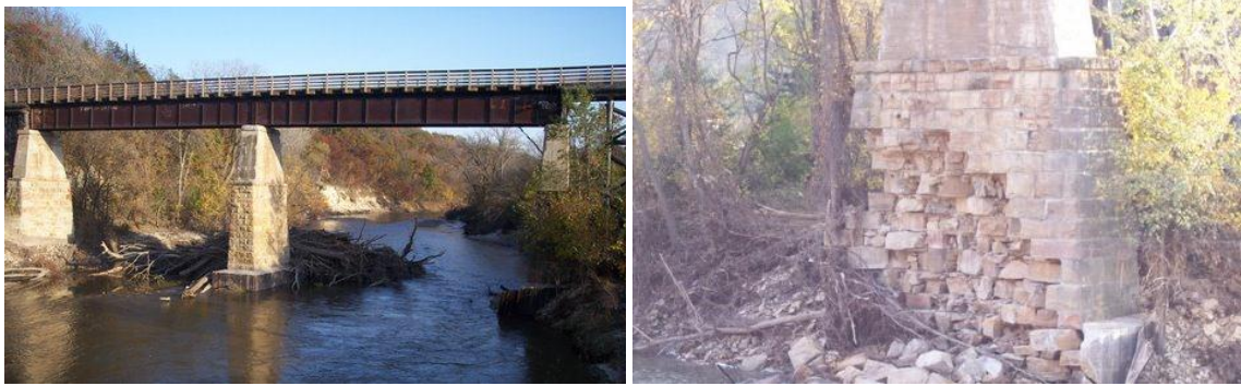
Figure 2.3: Bridge damage from Southern Minnesota flooding in October 2010 (Unknown, 2010)
