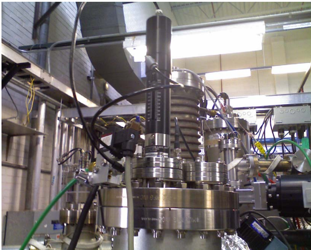
Photograph of Faraday Cup Assembly with Solenoid, (Center Left) and Faraday Cup Shaft (Center)
