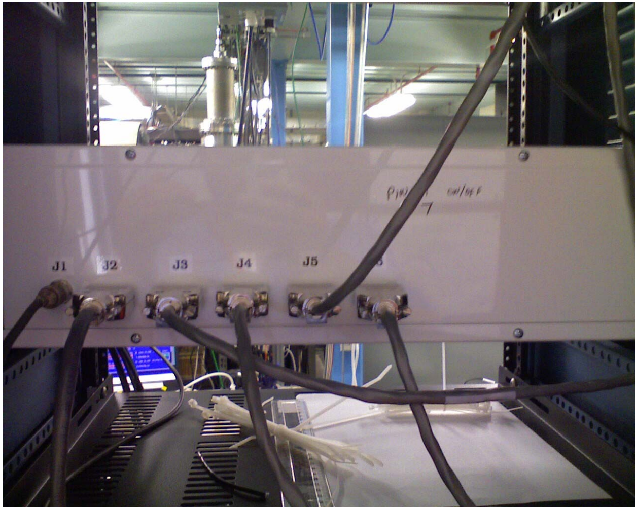
Figure 16. Rear View of the BPM Control System
