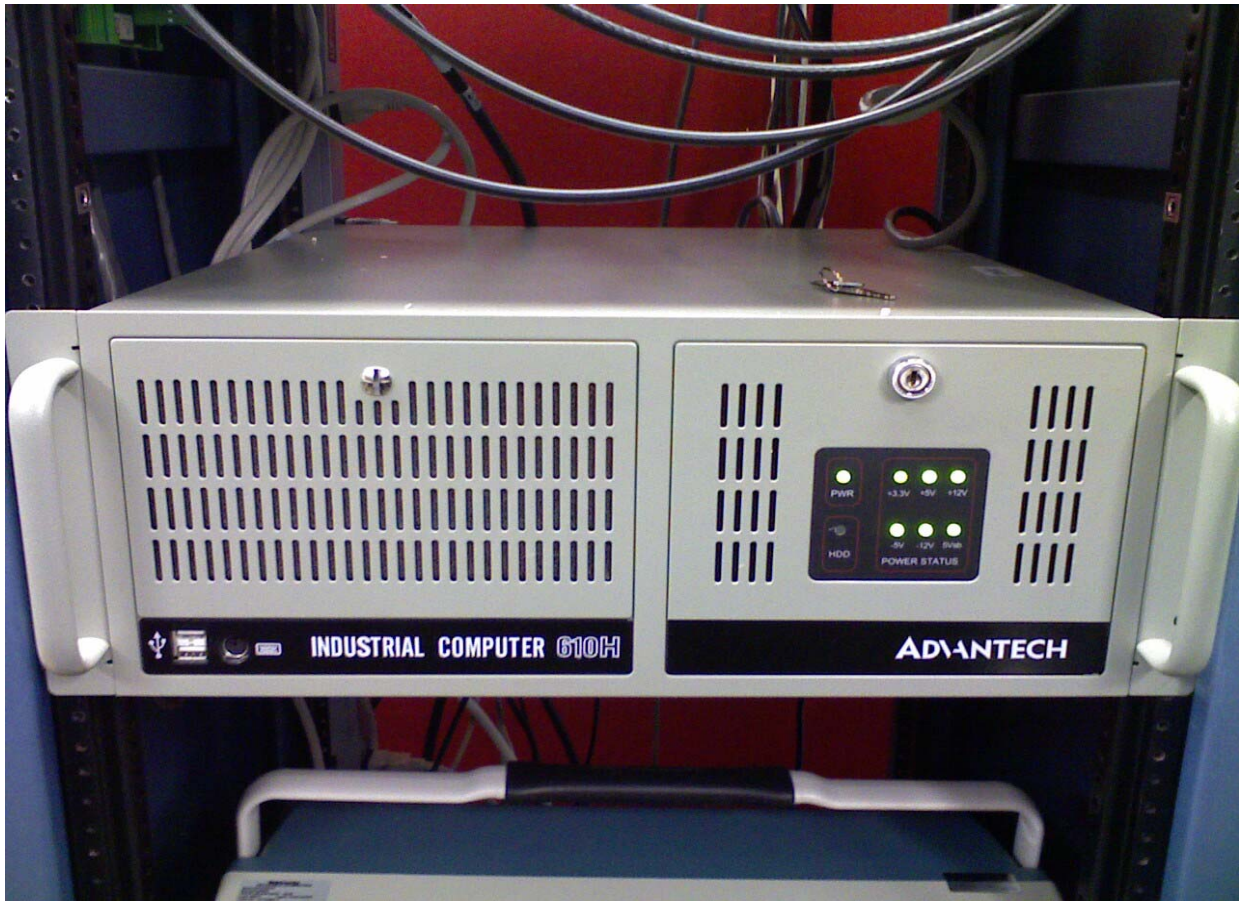
Figure 10. The New Industrial Computer Used in the Upgrade
