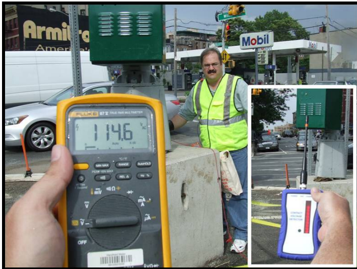
Figure 17. Energized traffic light base cause by direct contact with electric wiring
