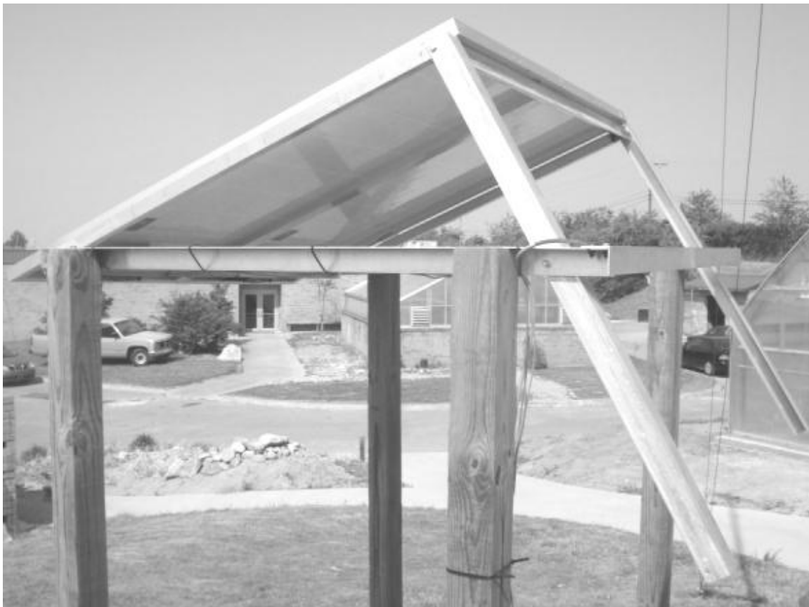
Figure 21. Adjustable Solar Panel Frame
