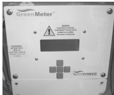
Figure 24. GreenMeter Power Management System
