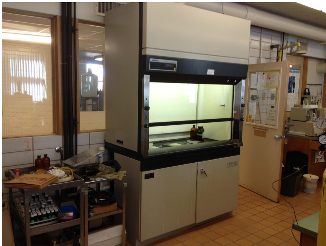
Figure 31. Environmental Health Sciences Lab Fume Extraction Hood
