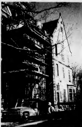
The renovation of Searles Science Building is expected to be completed by the fall of 1999. (Sherri Kies / Bowdoin Orient)
